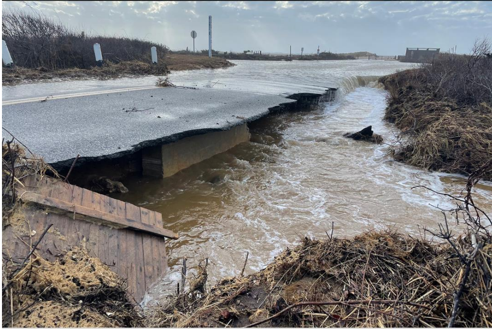
A culvert along Atlantic Drive in Edgartown failed, closing the road indefinitely.
