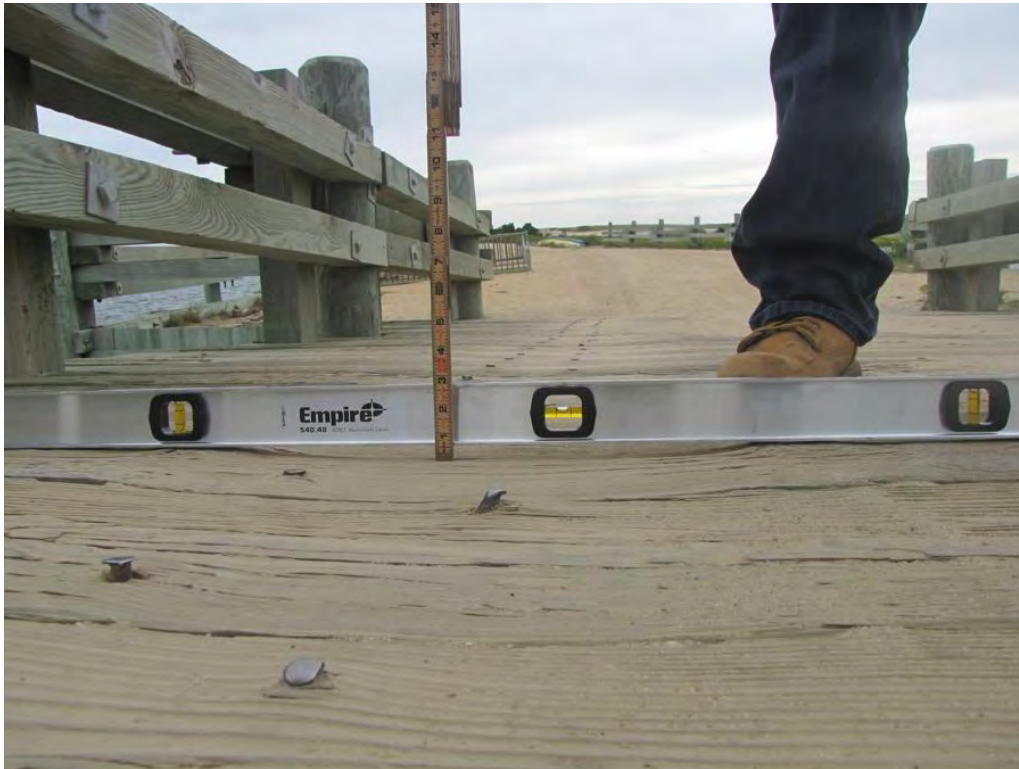
Photo 3: Close up of previous photo. Rutting and nails protruding up to 3/4"
