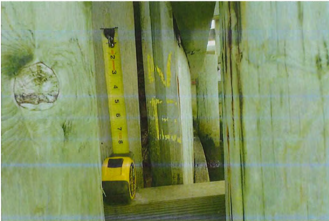
Photo 14: North corner of east abutment bulkhead looking south, bulging/bowing & gap w/ wingwall bulkhead.
