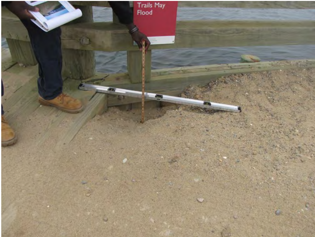
Photo 11: SW approach isolated sinkhole 2' W by 3' L by 1' D
