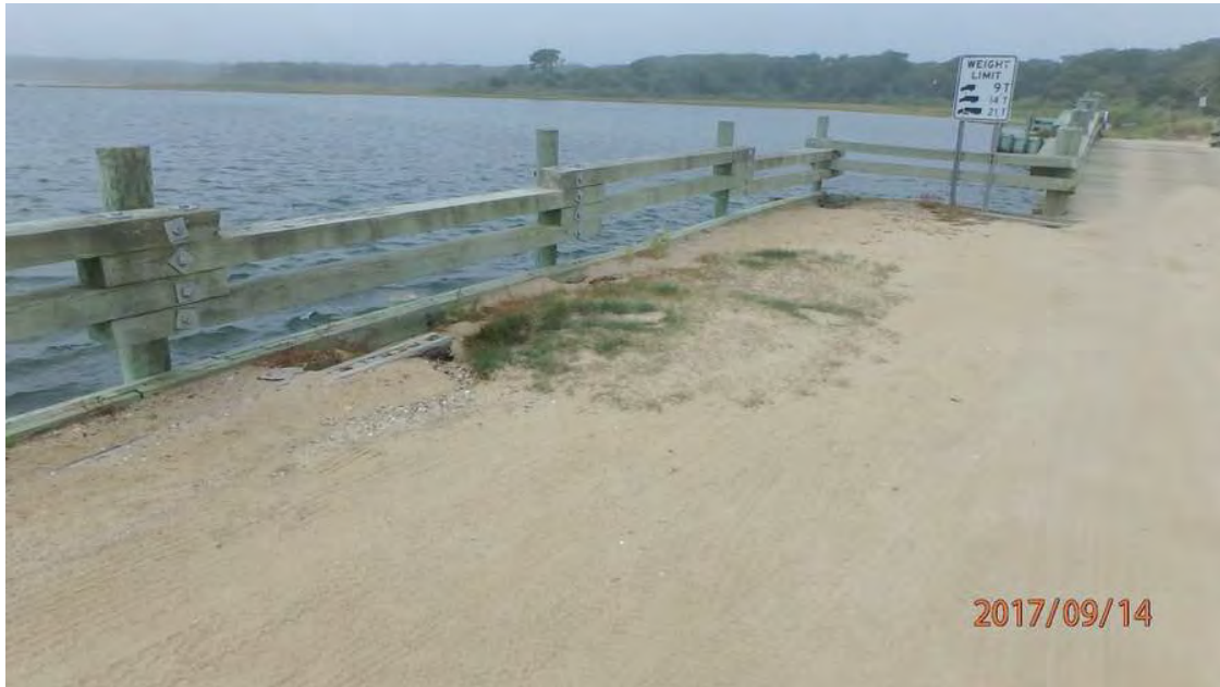
Photo 3: Southeast approach, minor erosion along retaining wall.
