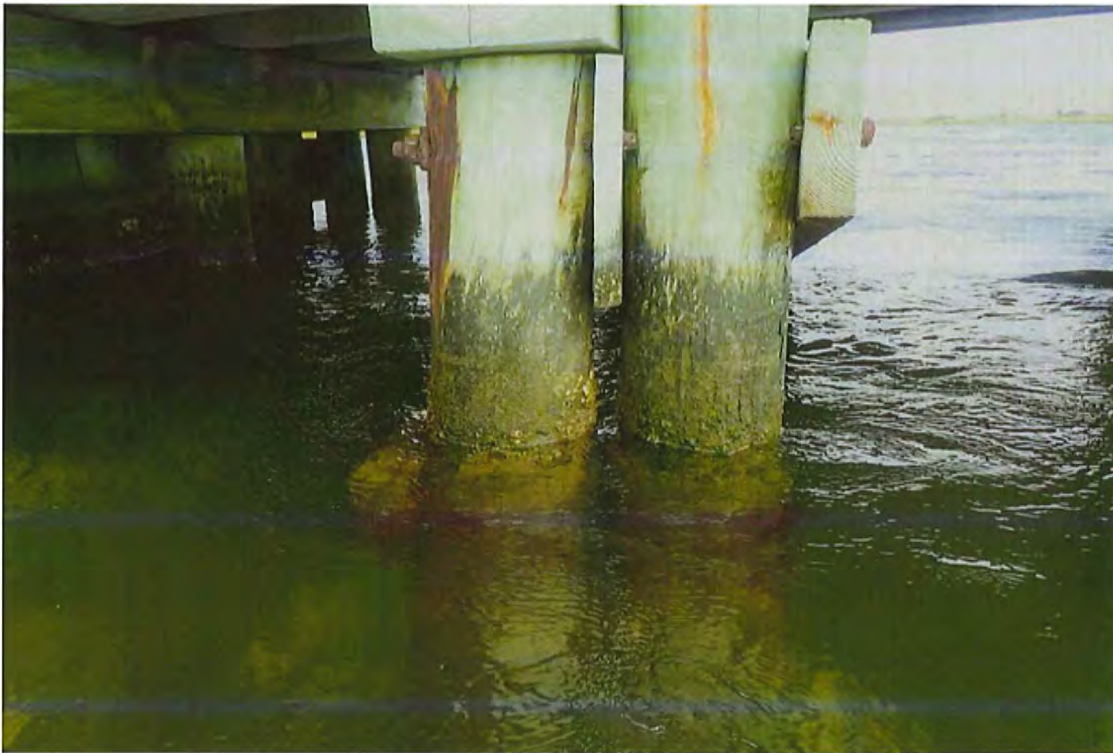
Photo 19: Bent 1 south piles, minor wane w/rust staining.
