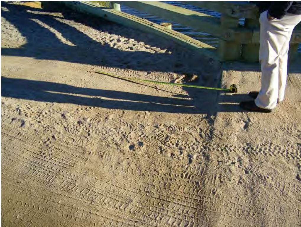
Photo 2: View west approach surface at span 1, 3' x 3' x 5" erosion/pothole.
