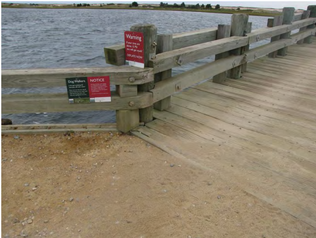
Photo 12: Overview of NW approach. Area has been filled in, since previous inspection
