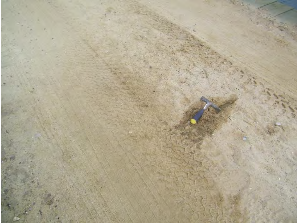
Photo 3: View east appro. and deck span #8, +/-2" deep sand debris.
