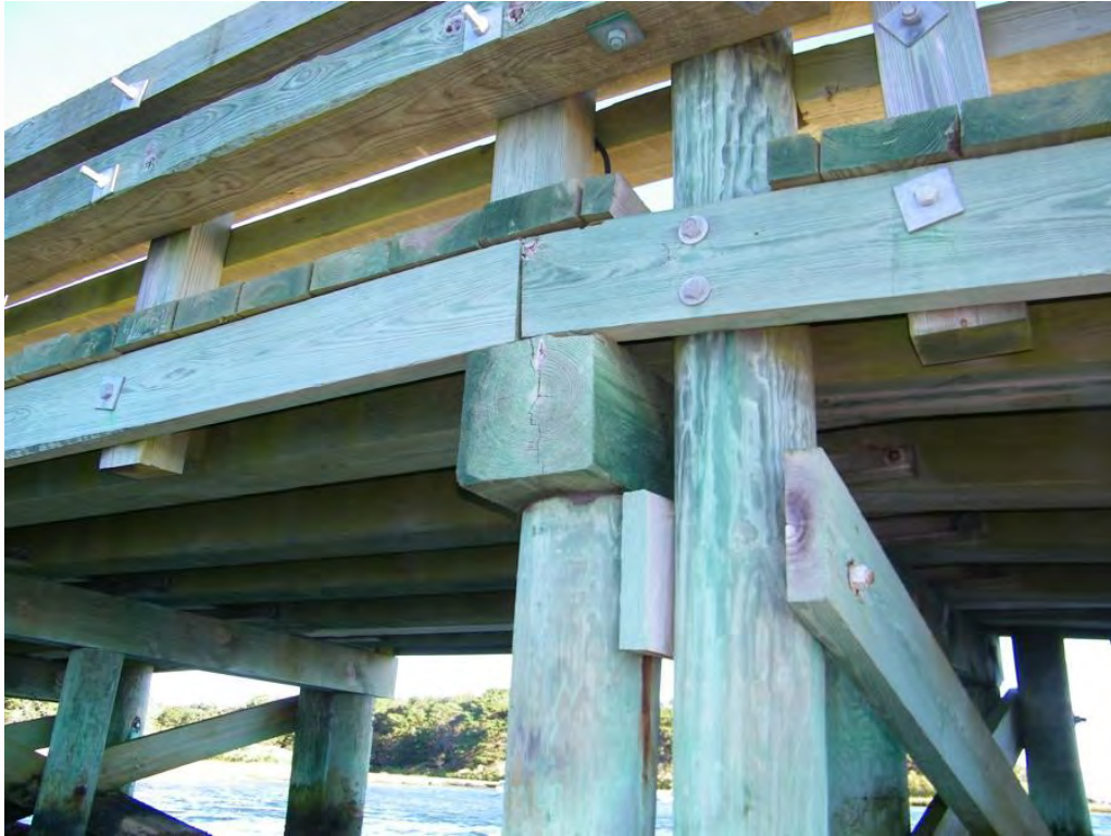
Photo 9: South end of timber pier cap 6, 1/8" wide splitting.
