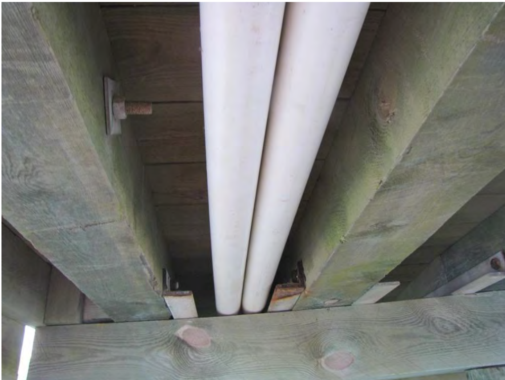
Photo 6: Typical utility bay
