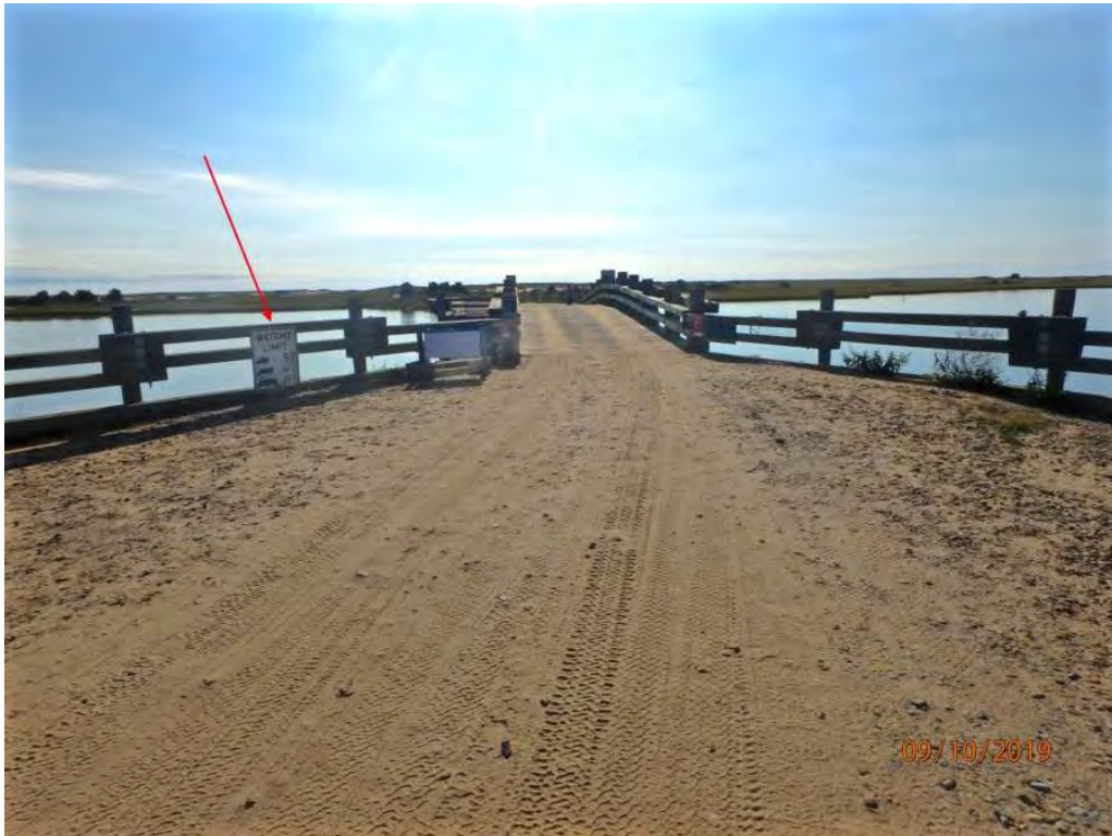
Photo 1: West approach, at-bridge weight posting sign installed at inadequate height
