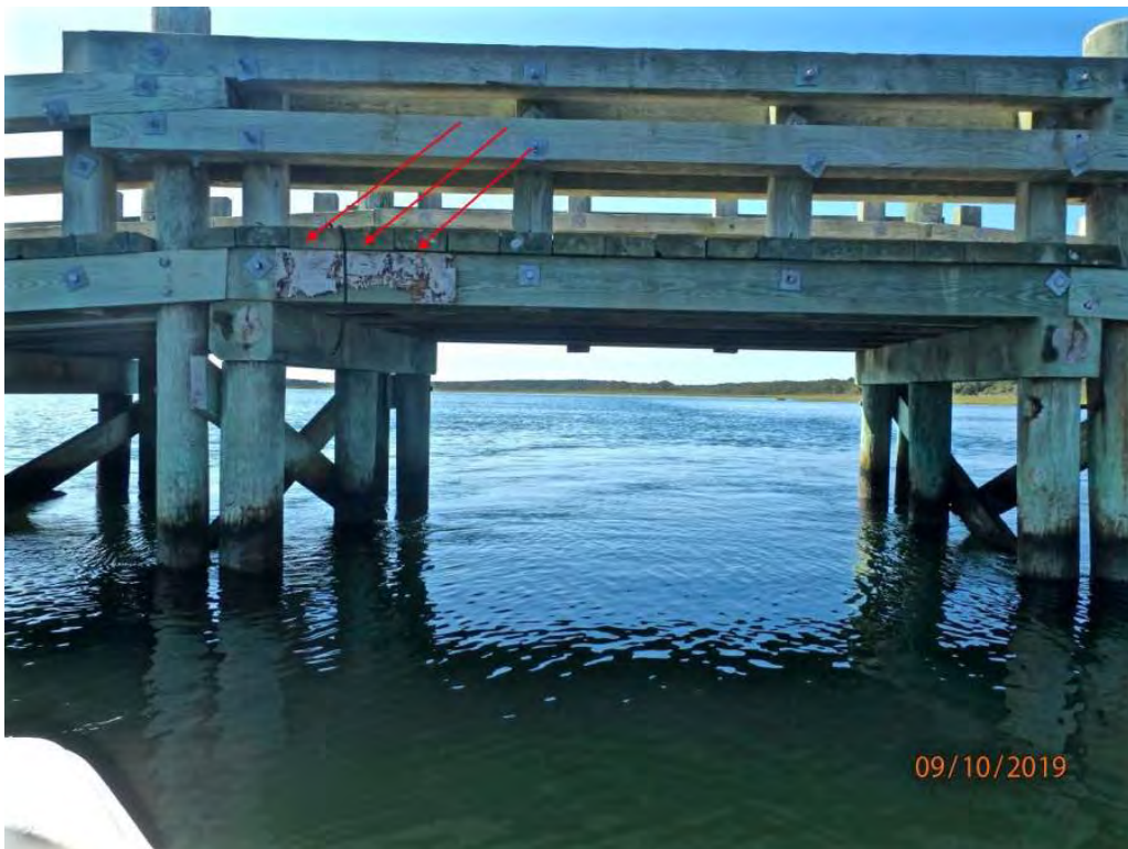
Photo 2: Span 5 north elevation, broken & missing navigation channel indicator sign
