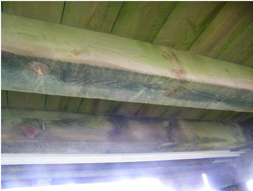
Photo 8: View underside typ. design/condition.
