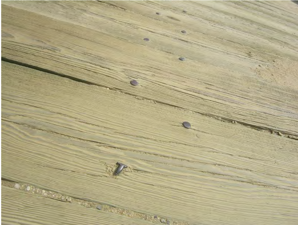
Photo 5: Two bent nails only.
