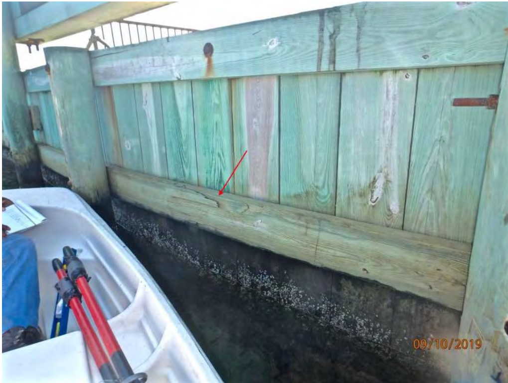
Photo 15: Northeast wingwall bulkhead between 1st & 2nd piles from west, split in middle wale
