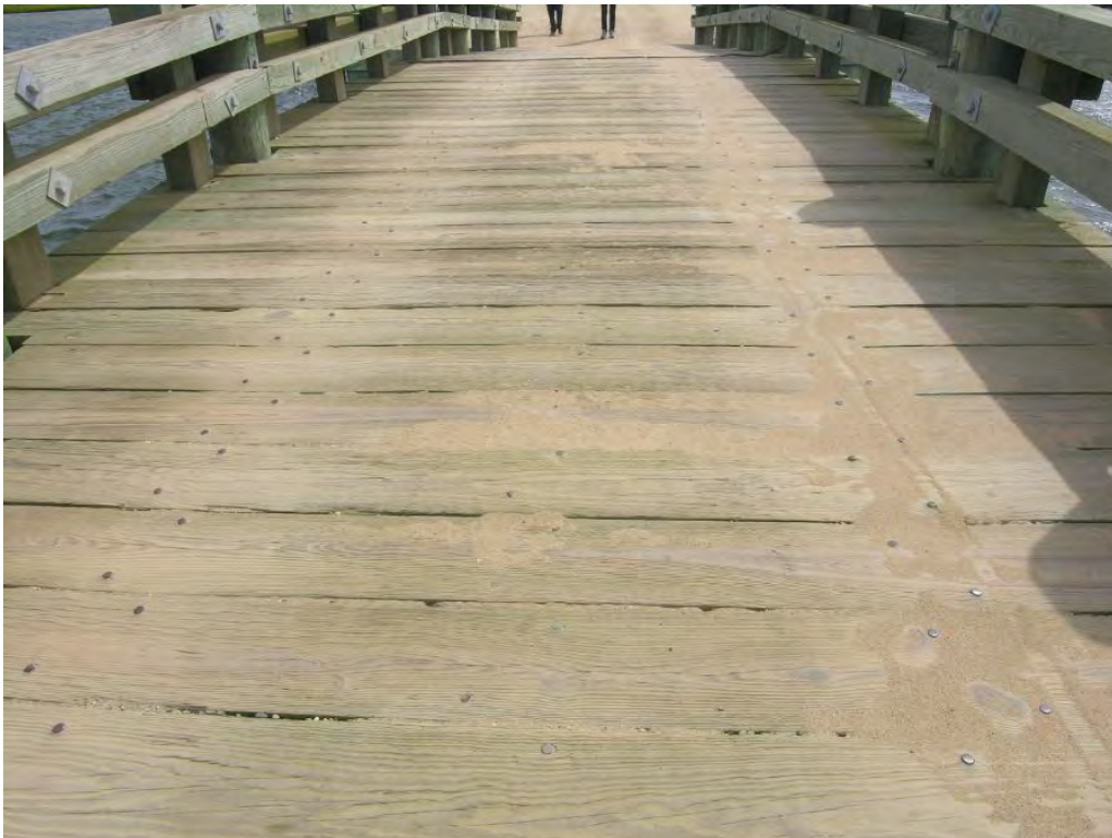
Photo 4: Timber wearing surface abrasion.
