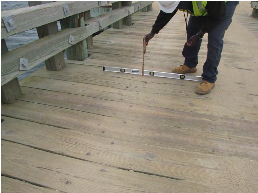
Photo 2: Overview of rutting
