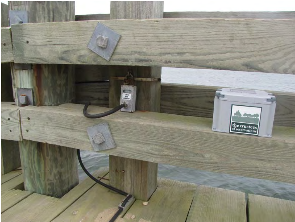
Photo 22: Overview of ADT counter. Previous and existing counter to the left (Count reads 37,668). New counter to the right, not connected up yet
