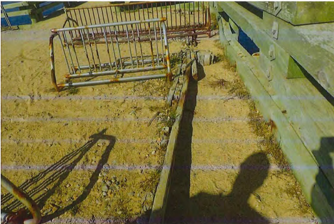
Photo 16: Northeast wingwall bulkhead at first tieback from west, bulging/bowing w/ gaps between sheathing & wales.
