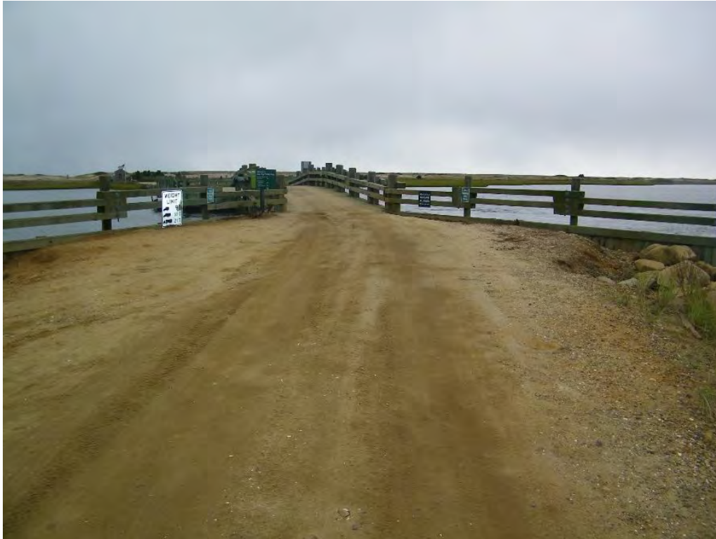
Photo 1: West at bridge weight posting sign.
