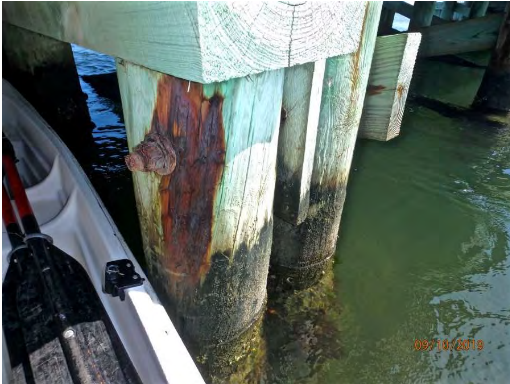
Photo 19: Bent 1 south piles, minor wane w/ rust staining
