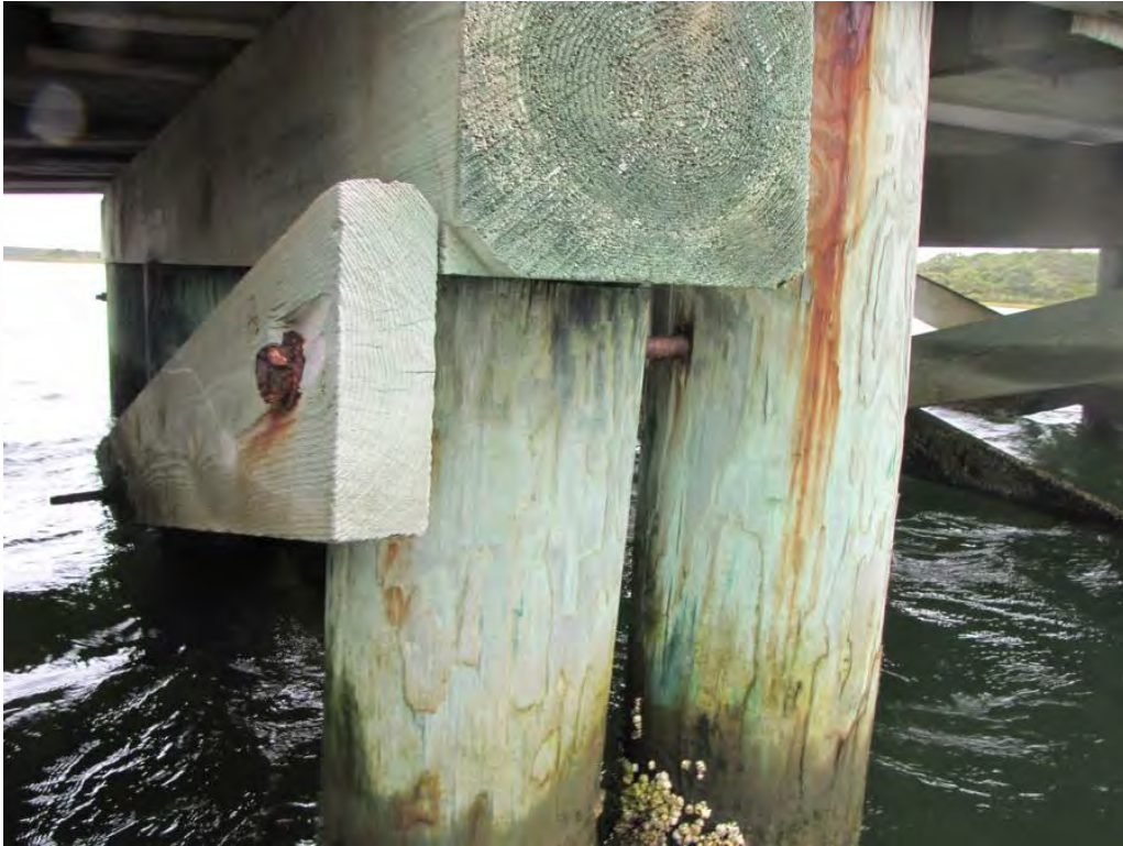
Photo 19: North bent fastener, isolated head of bolt starting to mushroom
