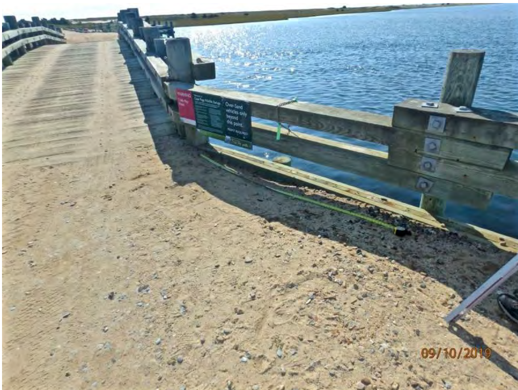
Photo 6: Southwest immediate approach roadway, corrective action taken since last inspection only minor erosion remains
