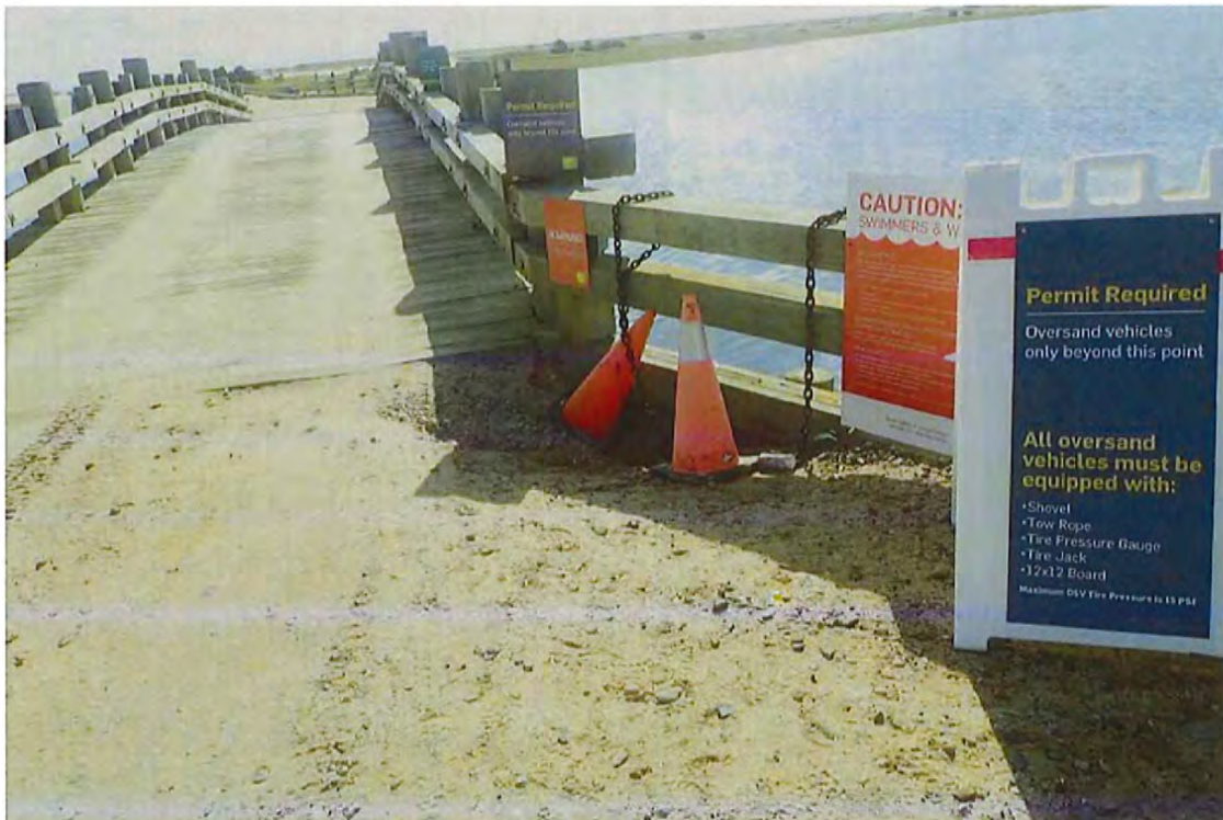
Photo 6: Southwest immediate approach roadway, erosion hole.
