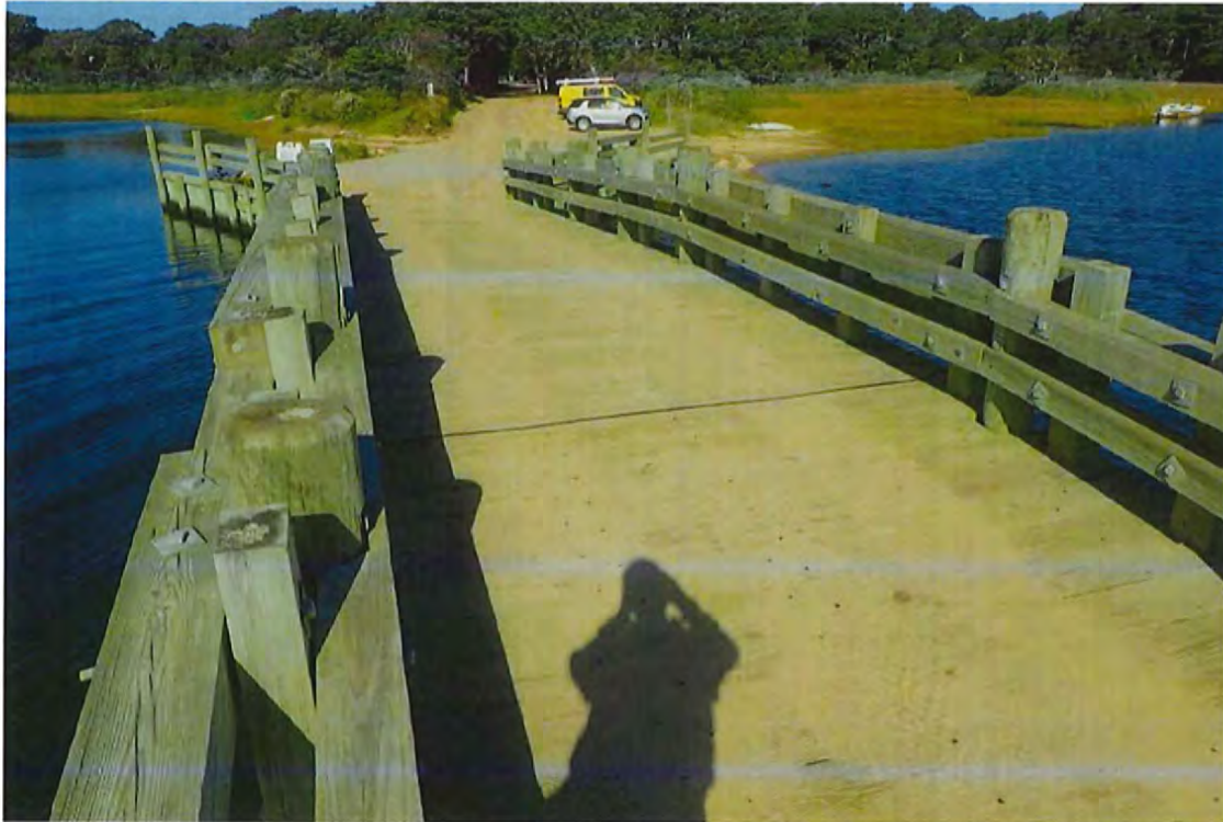
Photo 3: General wearing surface looking west, sand accumulation in abraded wheel paths.
