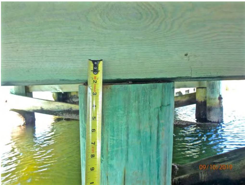
Photo 18: Bent 2 center pile east face, irregular cutoff w/ gap between cap
