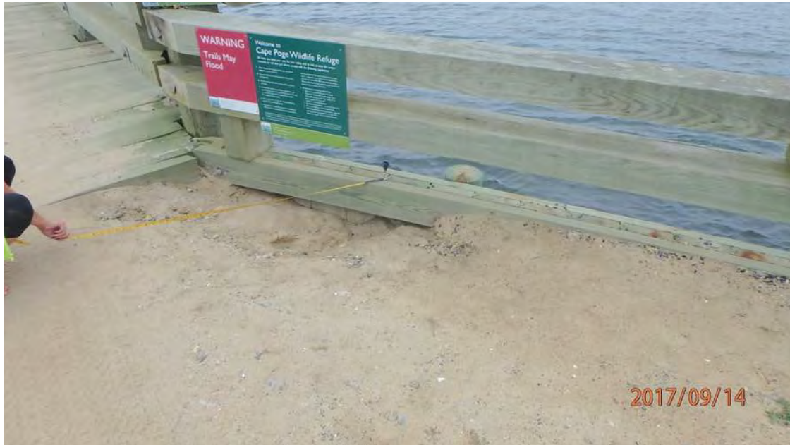
Photo 1: West approach, southwest corner erosion hole 7' x 2' x 10".
