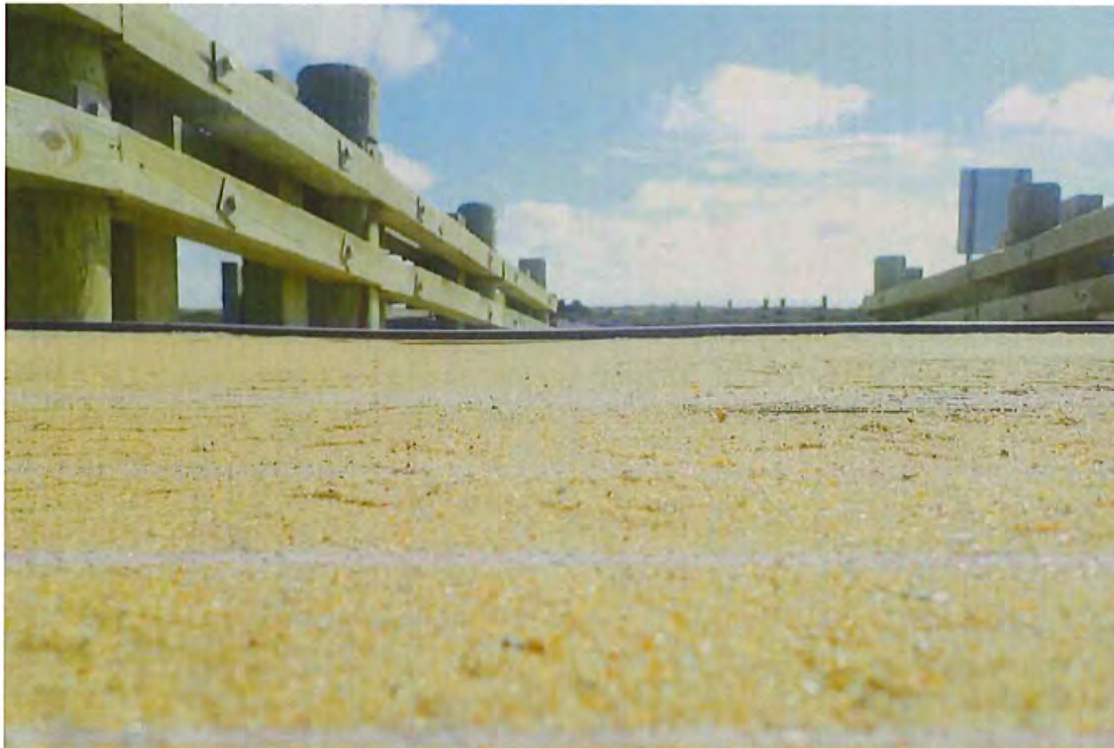
Photo 4: North wheel path looking east (Level @ Bent 4), abraded wheel path w/ sand accumulation & protruding fasteners.
