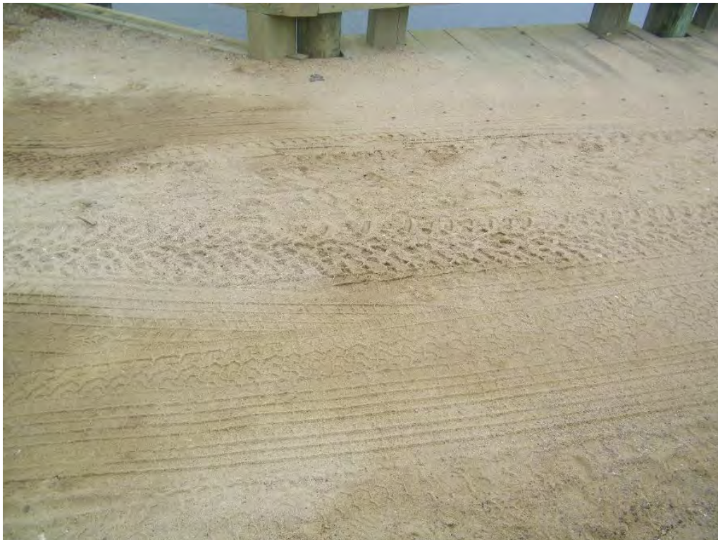
Photo 2: View west approx. and deck span #1, sand debris.
