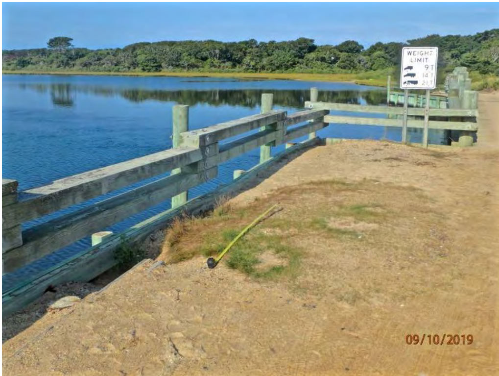
Photo 8: East approach along south wingwall bulkhead, correction action taken since last inspection moderate erosion remains
