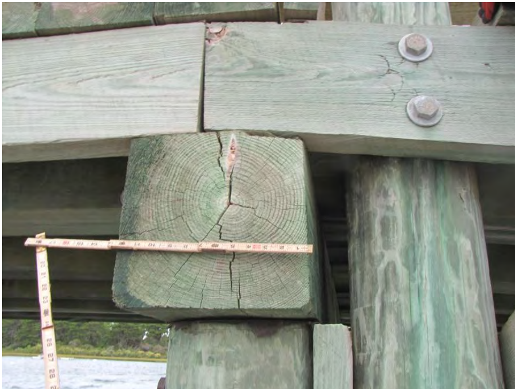
Photo 18: South end of timber pier cap 6. Isolated splitting up to 1/8" wide. No notable change
