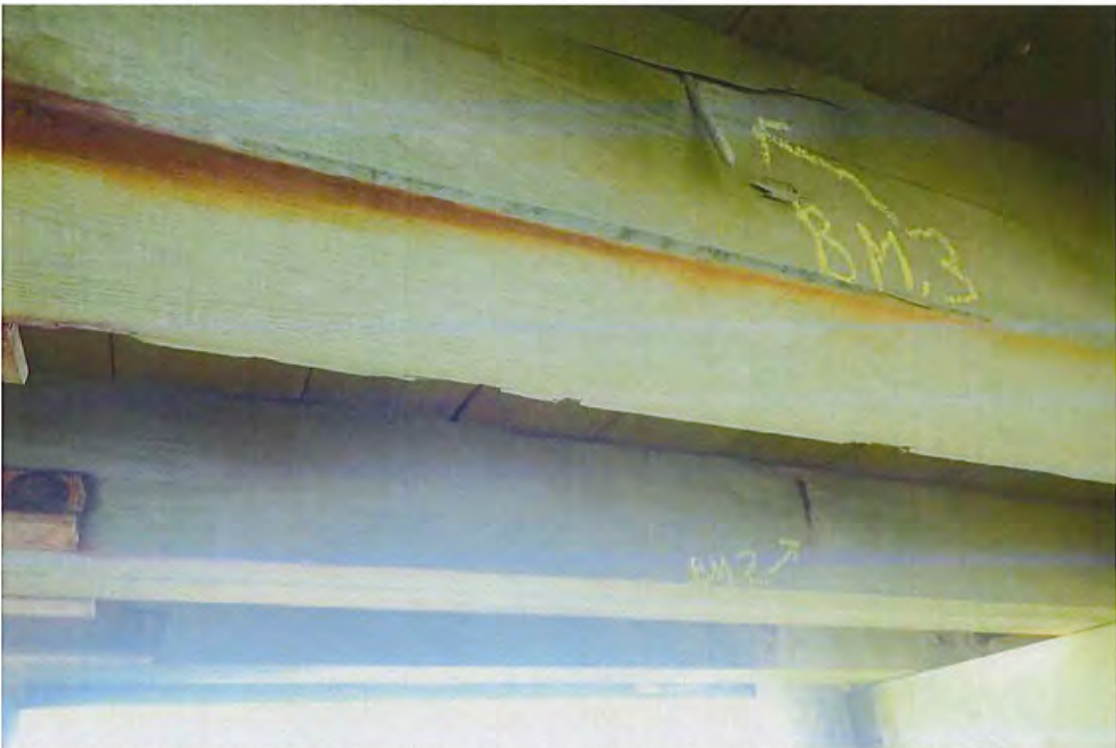
Photo 10: Span 2 Beam 2 north face, top edge split from misguided deck fastener.
