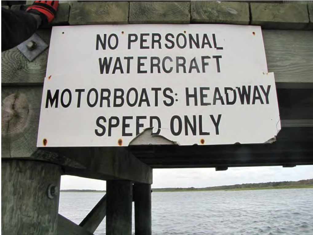
Photo 23: Sign over north face of navigation channel is damaged
