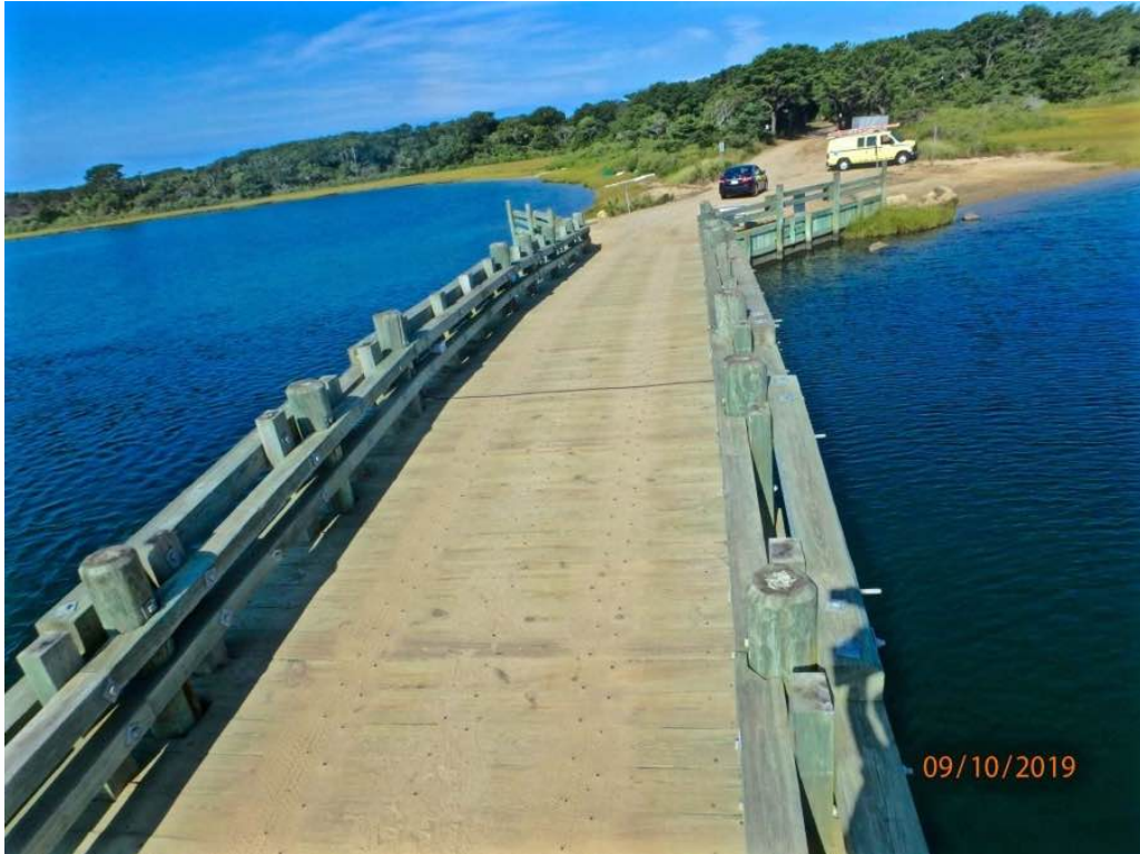
Photo 3: General wearing surface looking west, sand accumulation in abraded wheel paths
