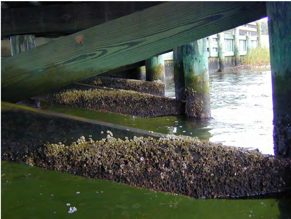
Photo 4: Build up of marine growth on all cross frames at high water mark down
