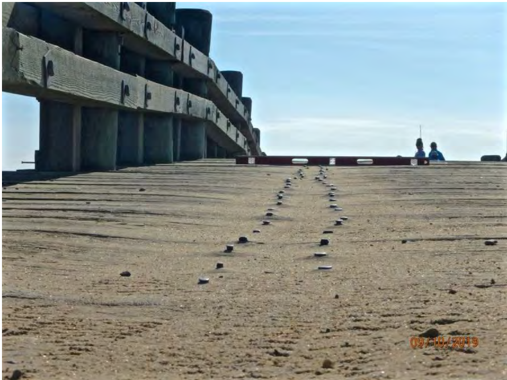
Photo 4: North wheel path looking east (Level @ Bent 4), abraded wheel path w/ sand accumulation & protruding fasteners
