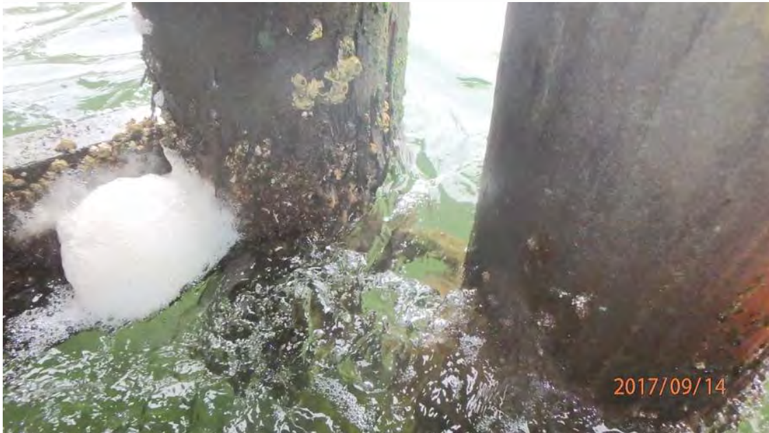
Photo 11: South end bent 7, southeast pile, notable abrasion/splintering in the tidal zone.
