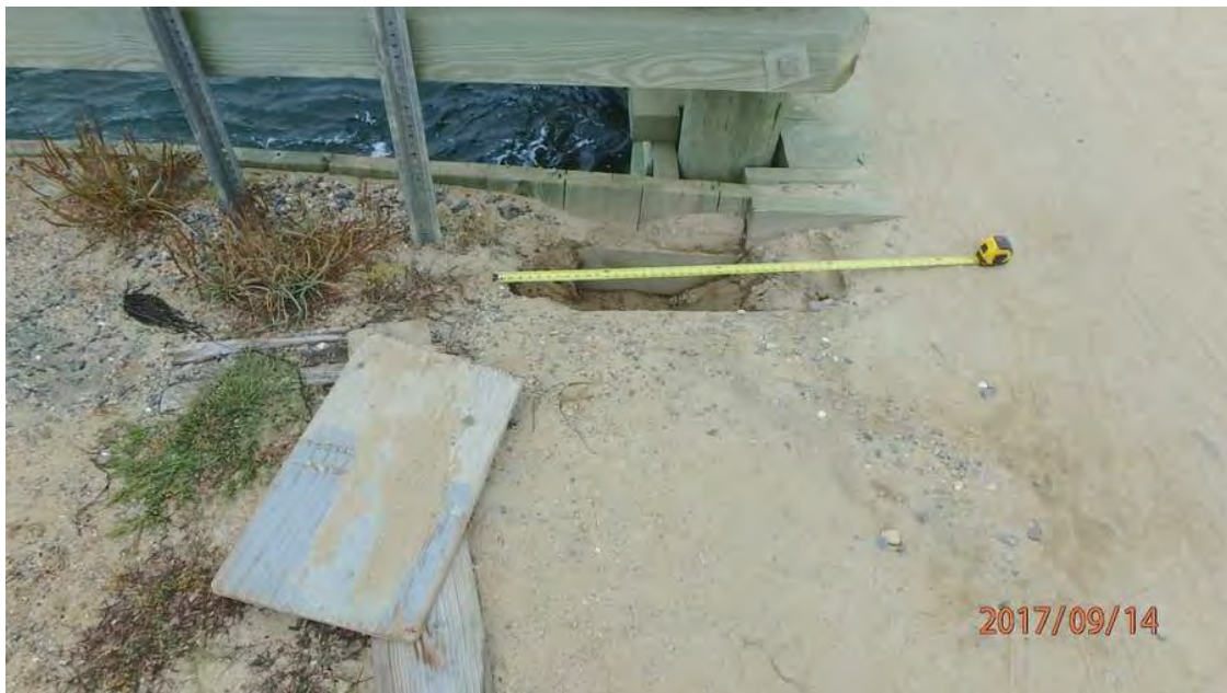
Photo 2: East approach, southeast corner erosion hole 3' x 20" x 14".
