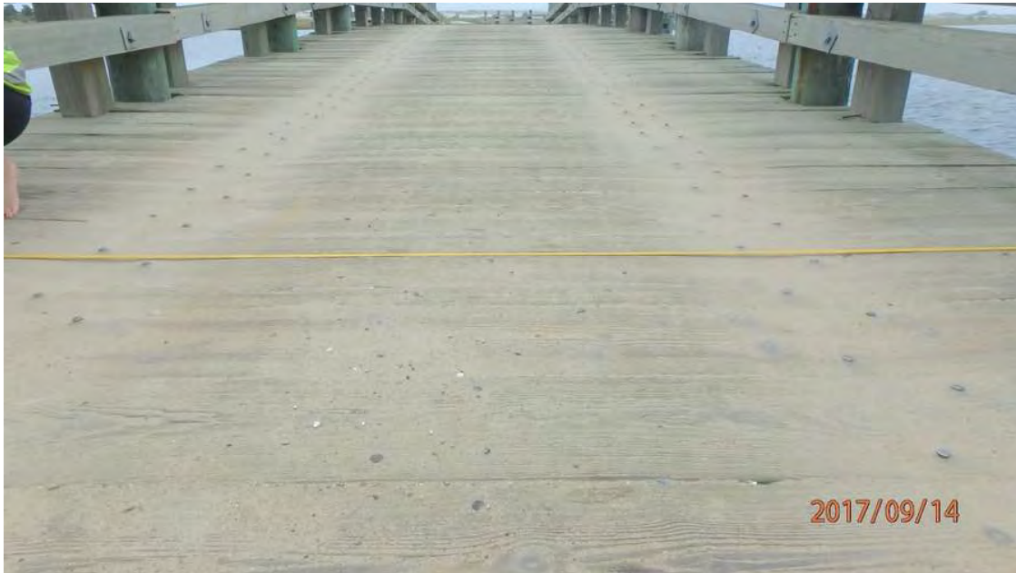
Photo 5: Close up view wearing surface rutting in the wheel path.
