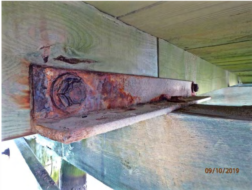
Photo 21: Bent 2 Beam 3 south keeper, corrosion to fastener hardware & angle
