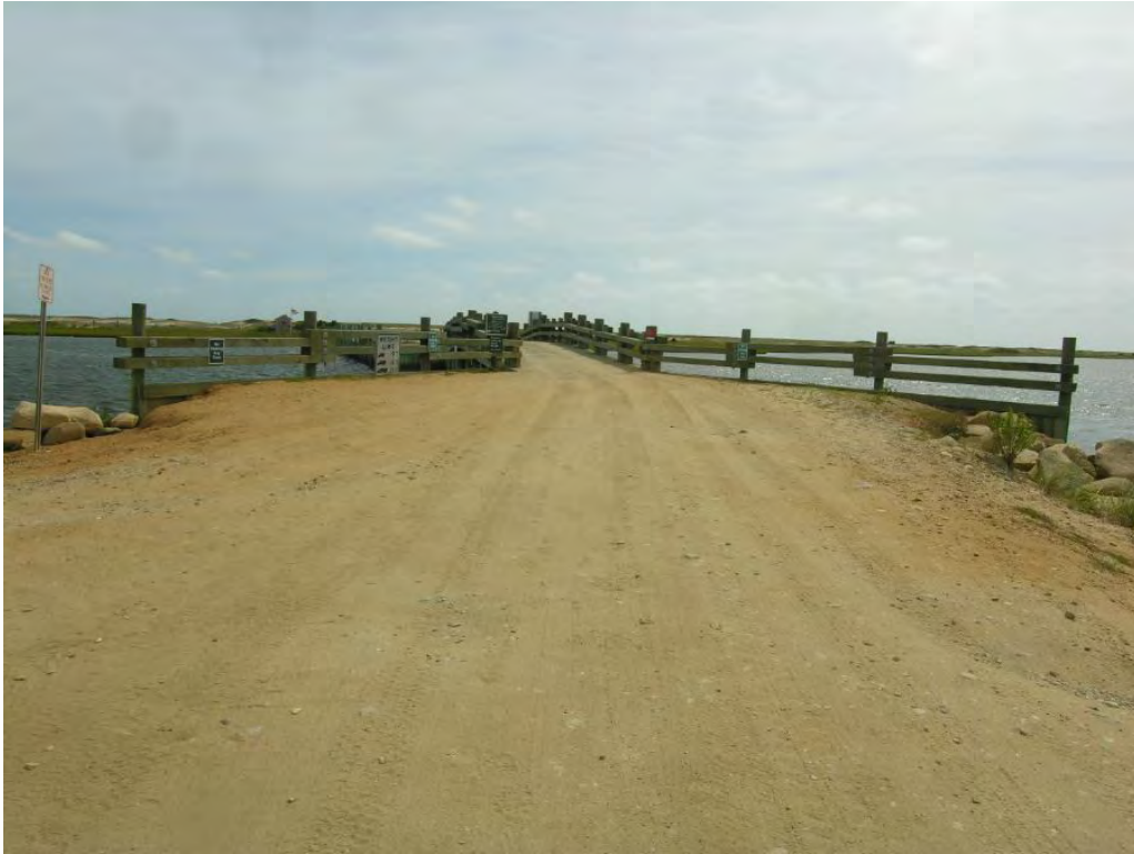
Photo 1: West at bridge weight posting sign.
