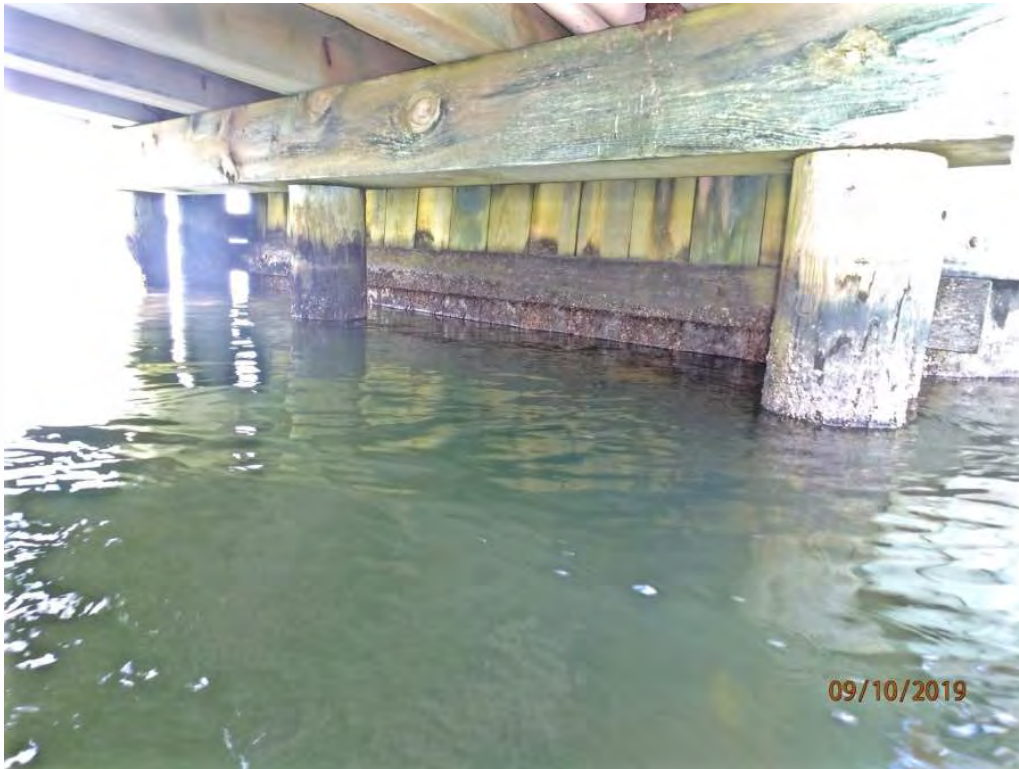
Photo 13: General view of west abutment bent & bulkhead, mildew staining & marine growth throughout
