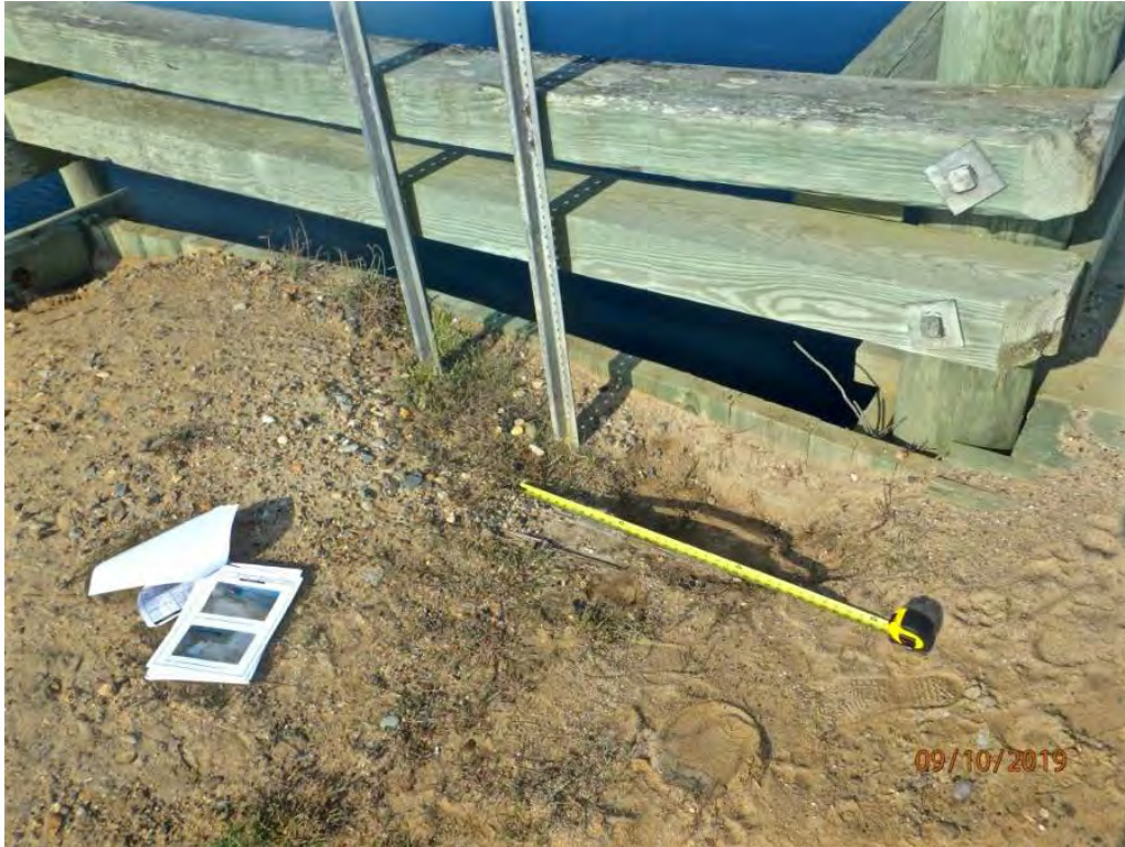
Photo 7: Southeast immediate approach roadway, corrective action taken since last inspection only minor erosion remains
