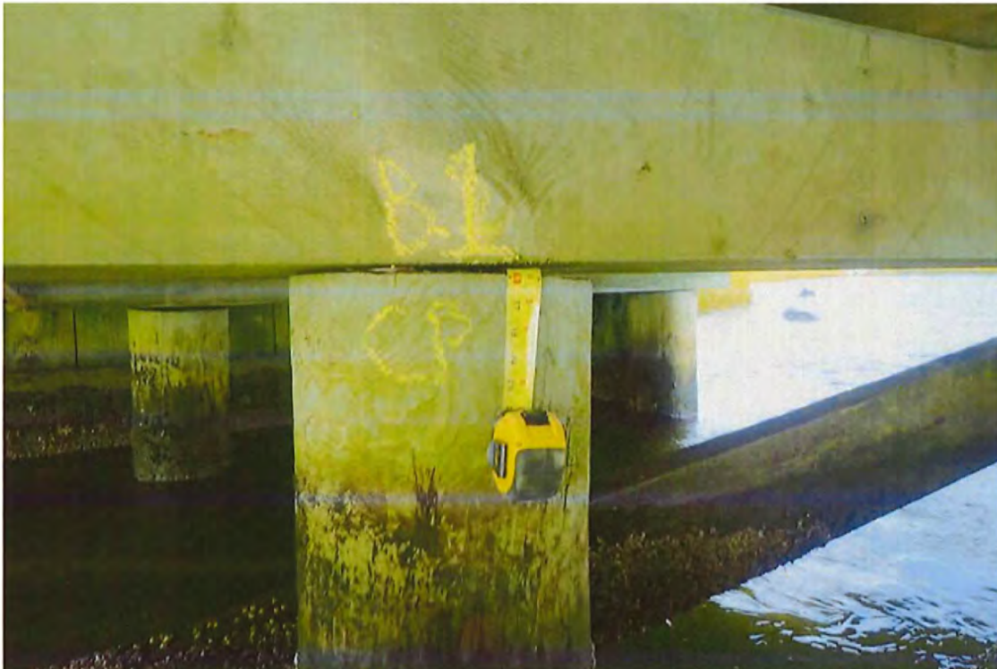
Photo 18: Bent 1 center pile east face, irregular cut off w/ gap between cap.
