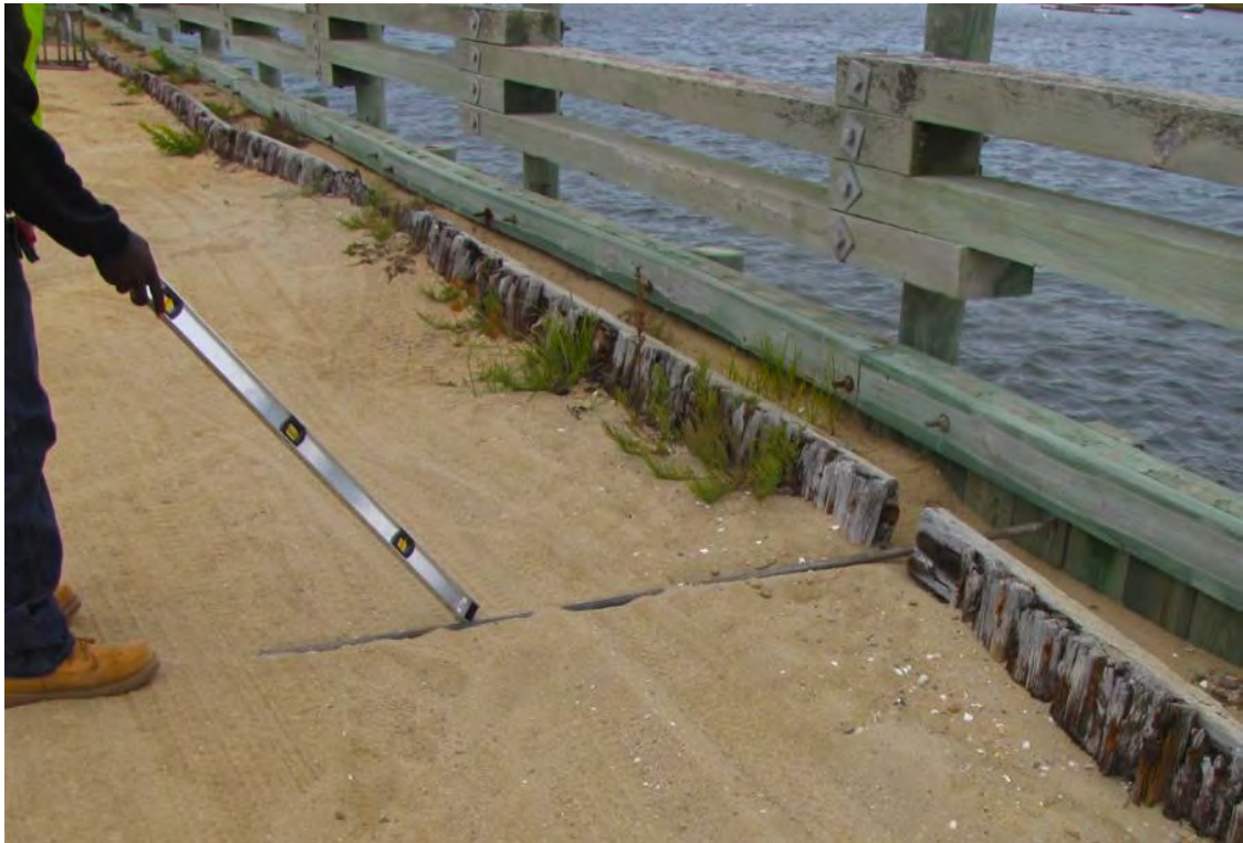
Photo 8: Close up of previous photo. Isolated exposed tie rod
