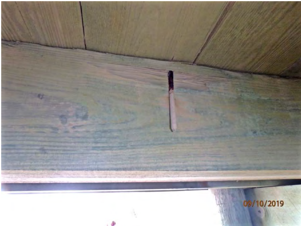
Photo 10: Span 2 Beam 2 north face, top edge split from misguided deck fastener
