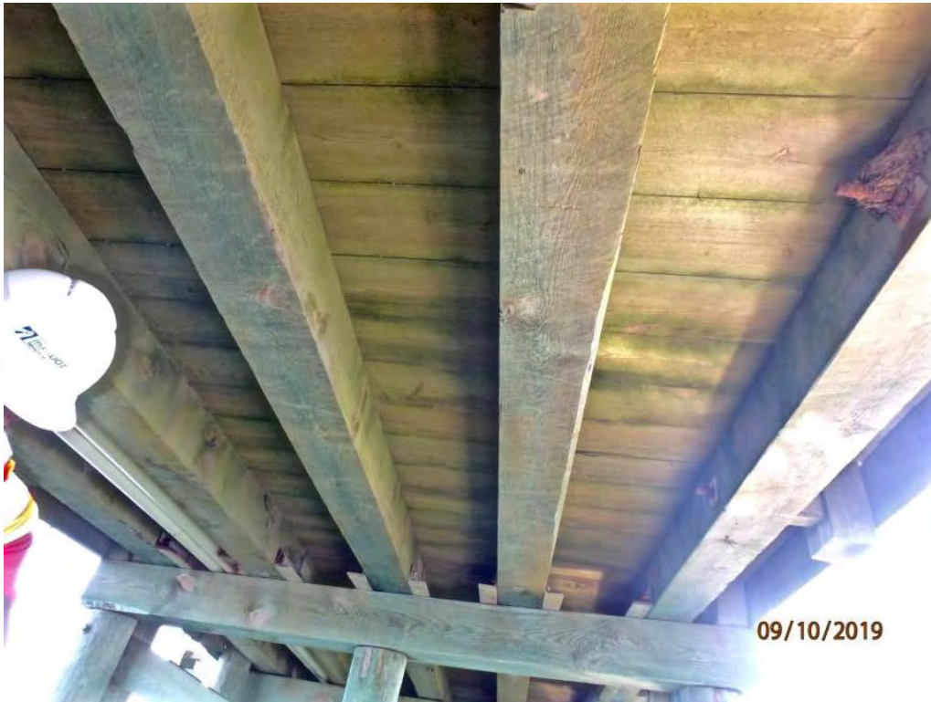
Photo 5: General underside Span 5 looking east, minor mildew staining throughout soffit
