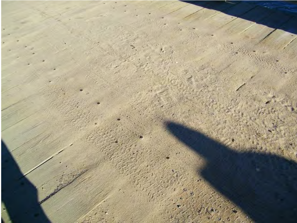
Photo 3: View east approach and deck span 8, 1/2" deep sand debris.
