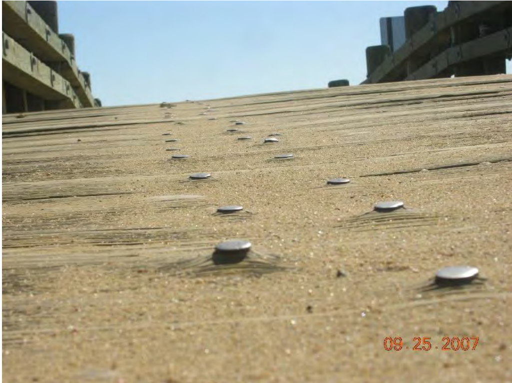
Photo 5: Wheel path wear
