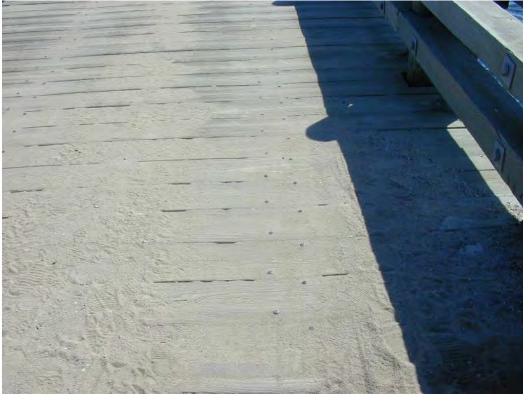
Photo 5: Roadway wheel path nails lifting.
