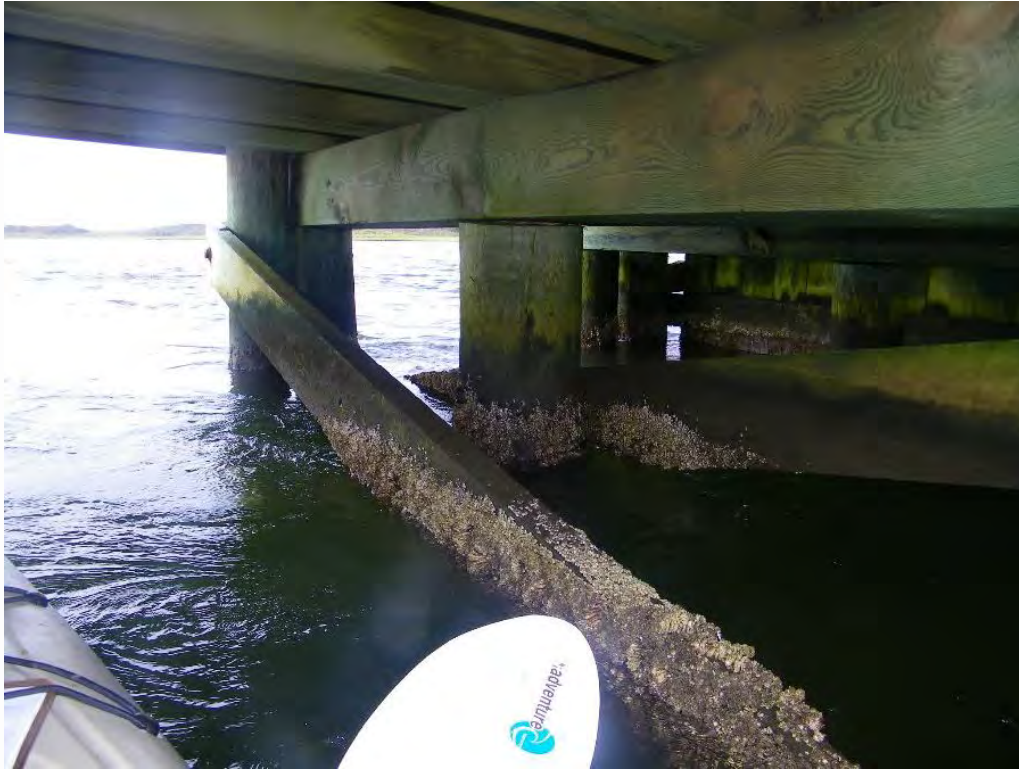
Photo 7: Pile/bent #2, east diagonal marine growth.
