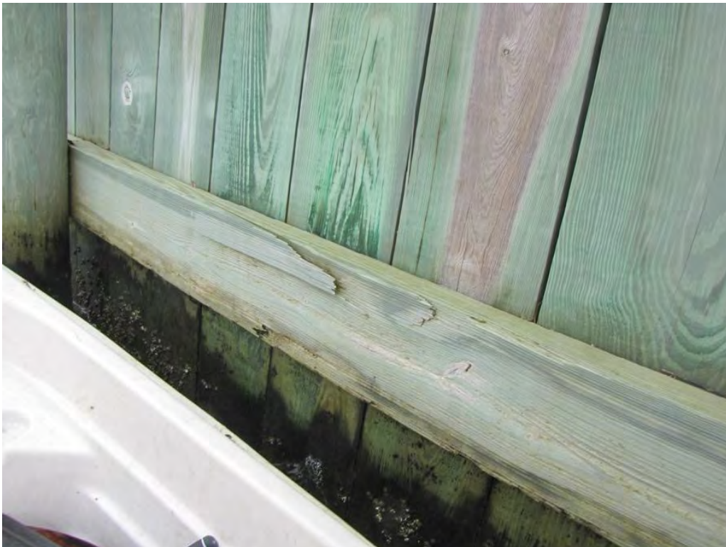
Photo 16: NE wingwall, isolated crack in lower timber
