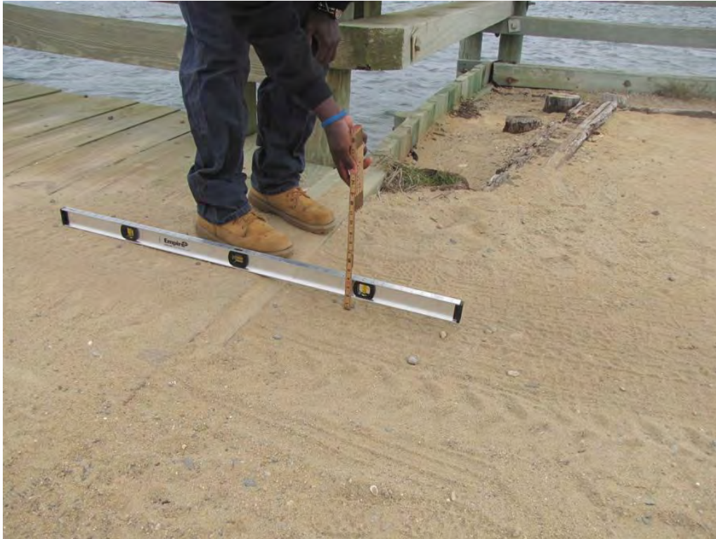
Photo 9: Typical settlement/rutting in wheel path at approach to bridge up 1-1/2"
