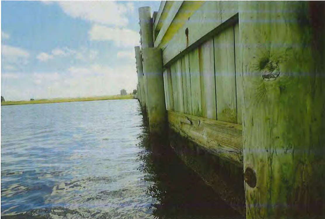
Photo 15: Northeast wingwall bulkhead between 1st & 2nd piles from west, split in middle wale.
