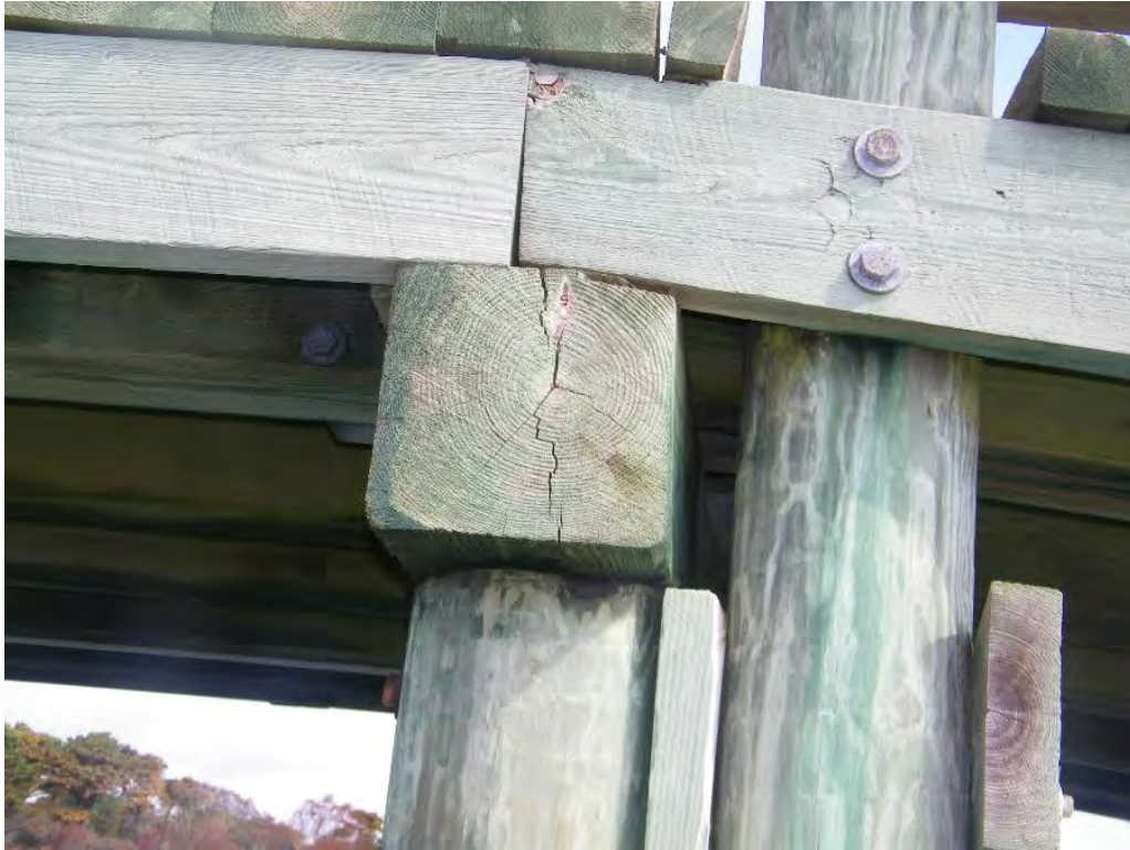
Photo 9: South end timber pier cap #6, +/-1/8" wide checking.
