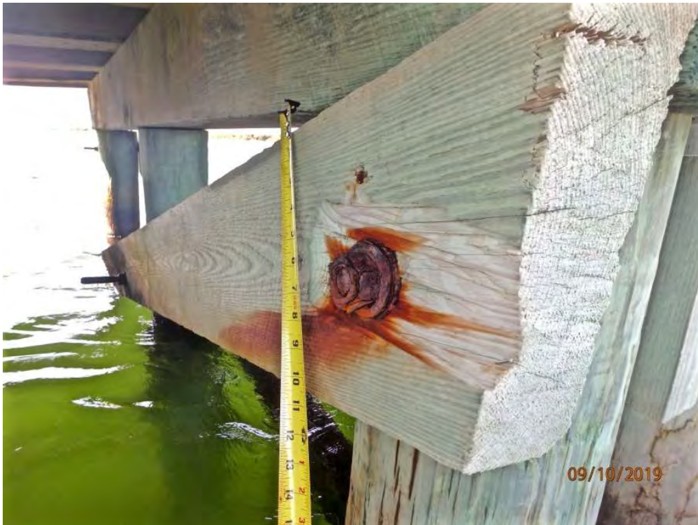
Photo 20: Bent 7 north end of east diagonal bracing, corrosion of fastener hardware
