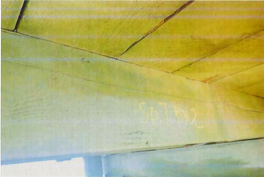
Photo 11: Span 7 Beam 2 south face, horizontal surface checking.
