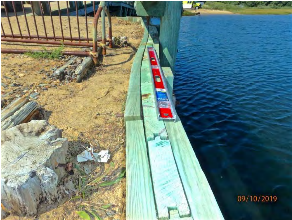
Photo 16: Northeast wingwall bulkhead at first tieback from west, bulging/bowing w/ gaps between sheathing & wales
