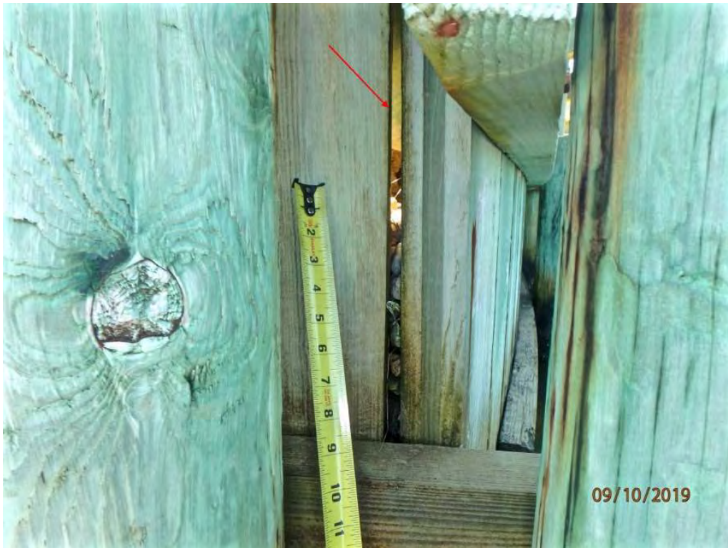
Photo 14: North corner of east abutment bulkhead looking south, bulging/bowing & gap w/ wingwall bulkhead
