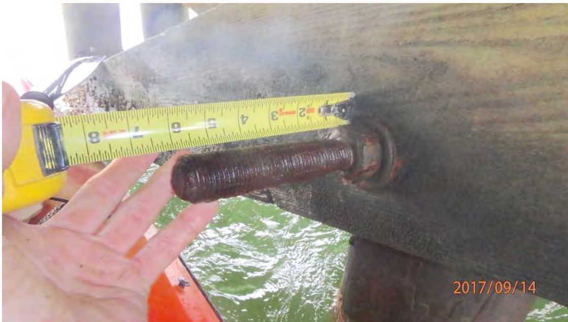
Photo 8: Common rusting fastening hardware conditions in the tidal zone.
