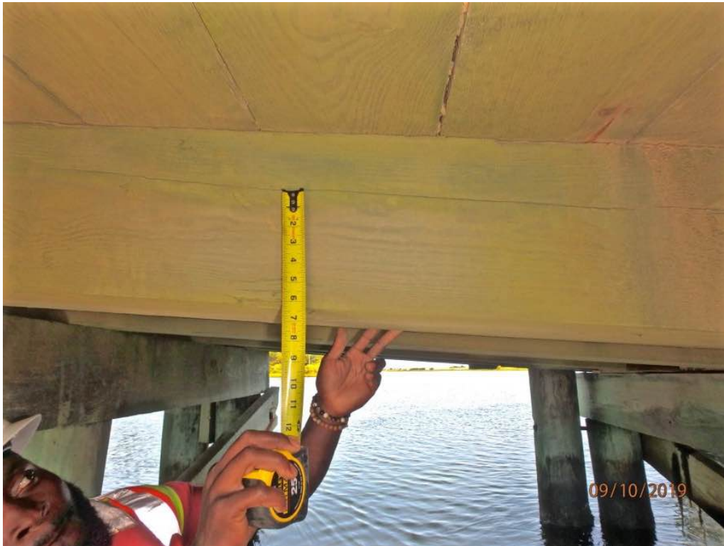
Photo 11: Span 7 Beam 2 south face, horizontal checking
