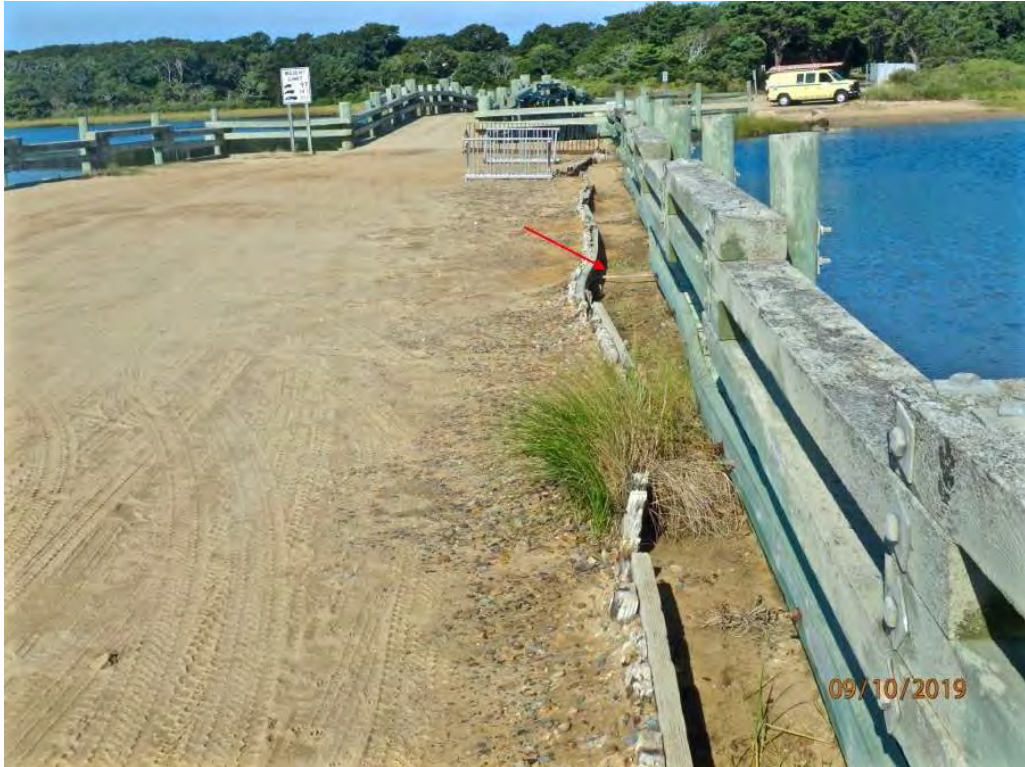
Photo 9: East approach along north wingwall bulkhead, erosion along abandoned bulkhead exposing tiebacks
