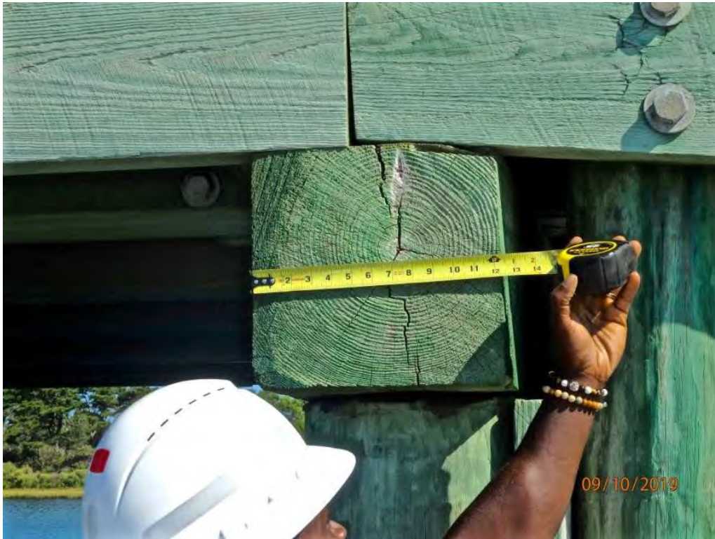
Photo 17: Bent 5 south face of cap, vertical end check
