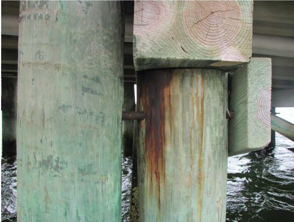
Photo 21: Some bolts showing some corrosion, scale, and start of section loss
