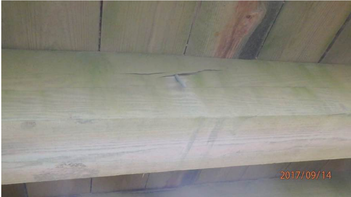
Photo 7: Scattered deck spikes puncturing side of beams.
