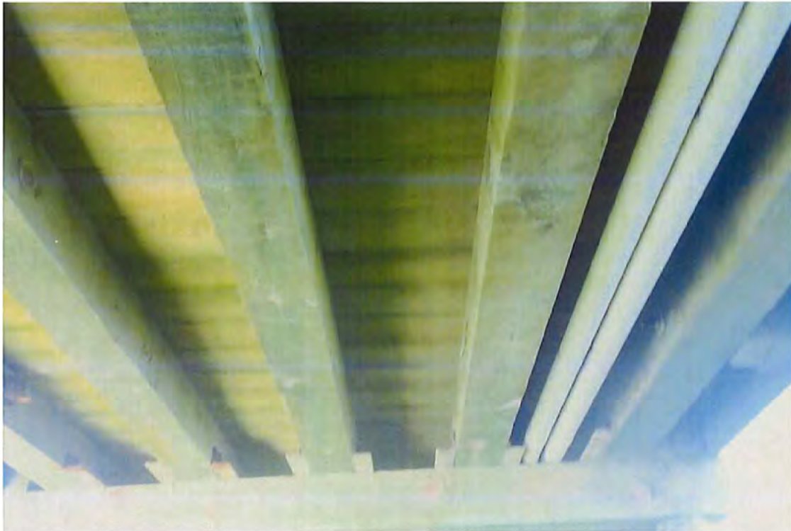
Photo 5: General underside Span 5 looking west, minor mildew staining throughout soffit.
