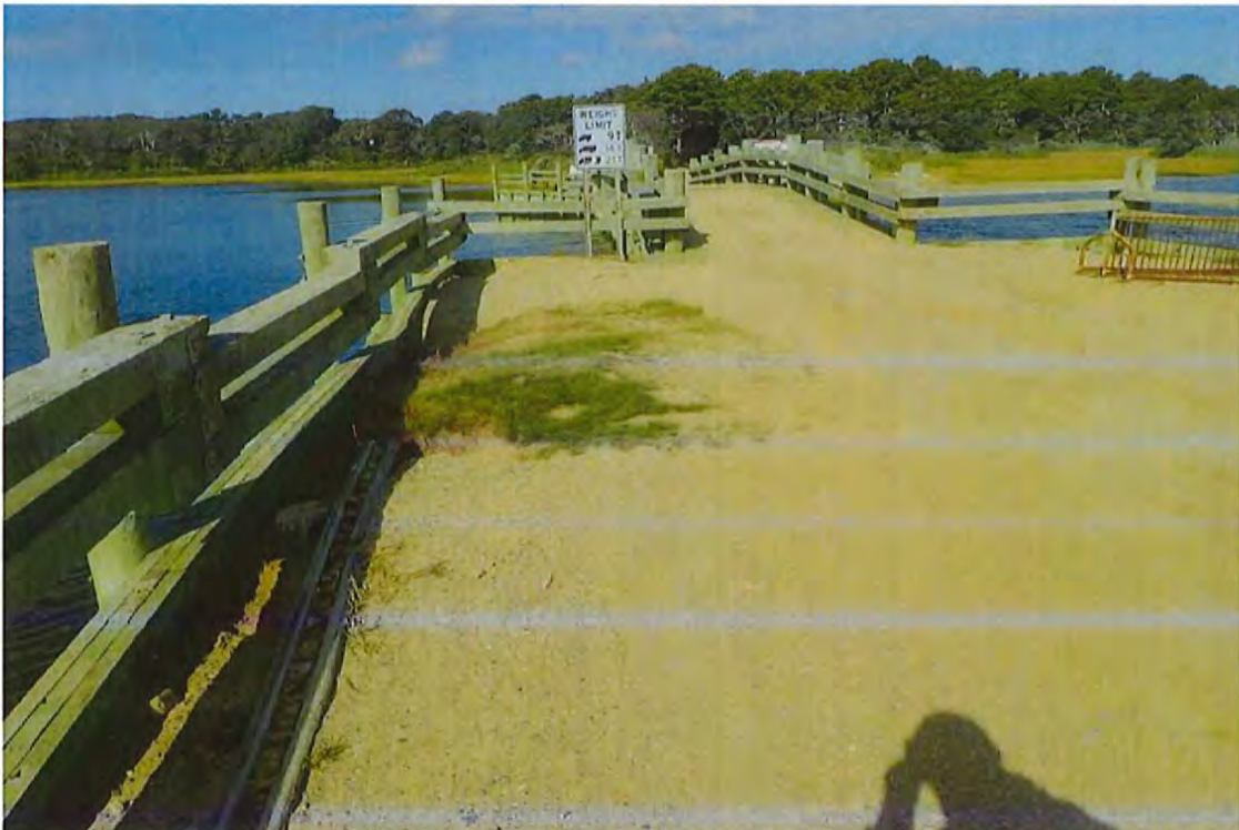
Photo 8: East approach along south wingwall bulkhead, moderate erosion.
