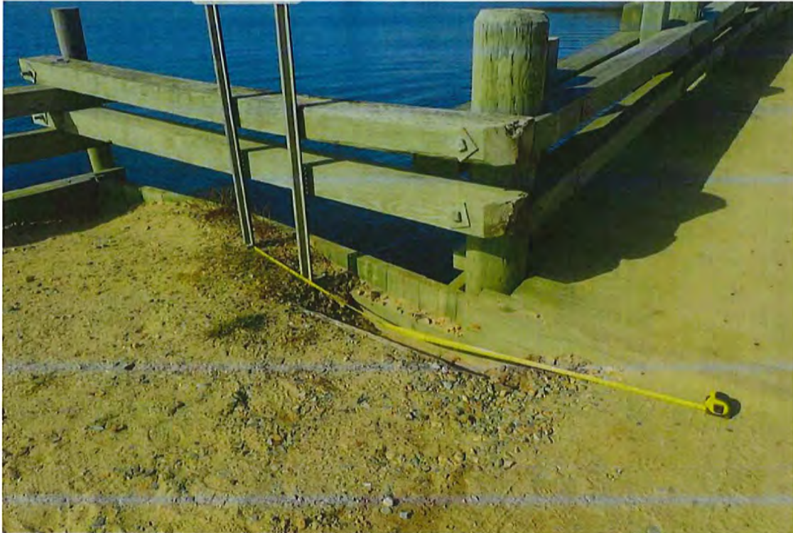
Photo 7: Southeast immediate approach roadway, erosion hole.
