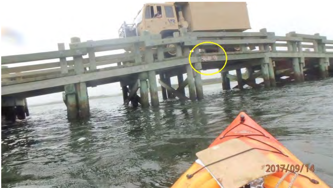
Photo 12: North elevation, channel sign missing, and truck traffic.
