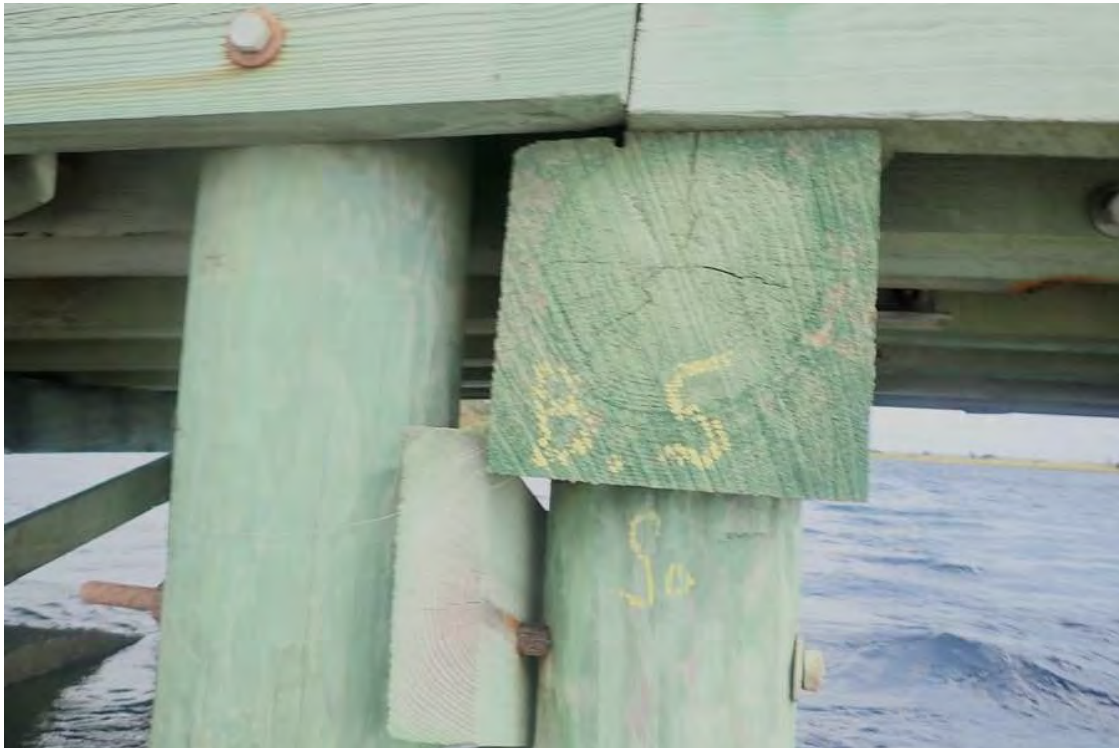
Photo 17: Bent 5 south face of cap, vertical end surface checks.
