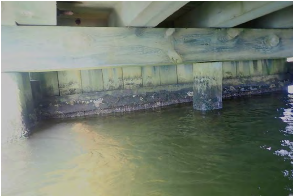
Photo 13: General view of west abutment bent & bulkhead, mildew staining & marine growth throughout.
