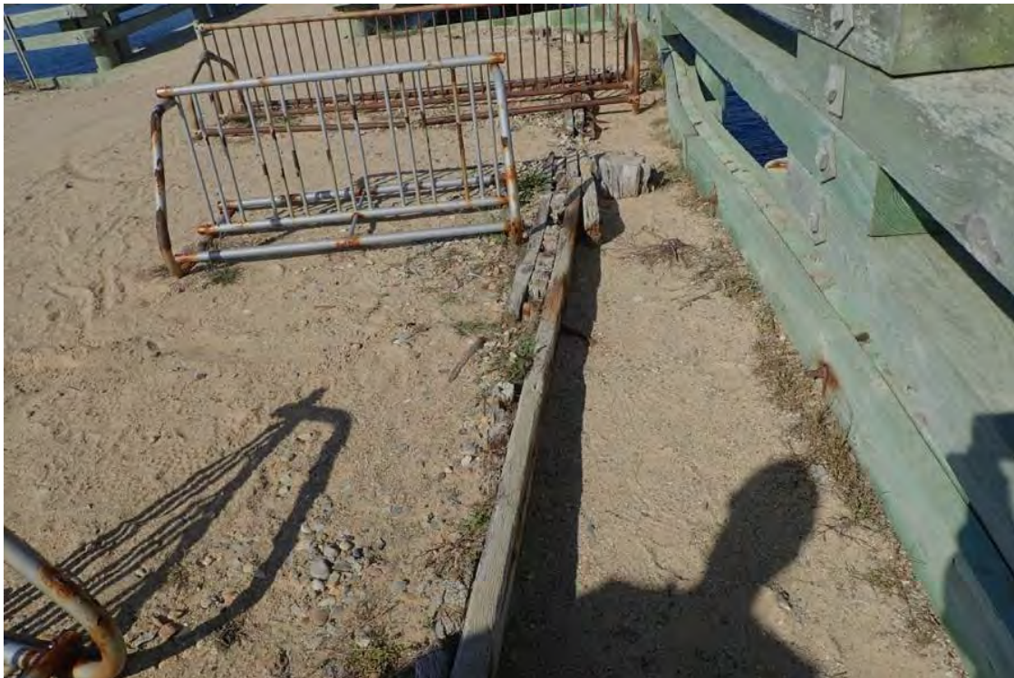
Photo 16: Northeast wingwall bulkhead at first tieback from west, bulging/bowing w/ gaps between sheathing & wales.
