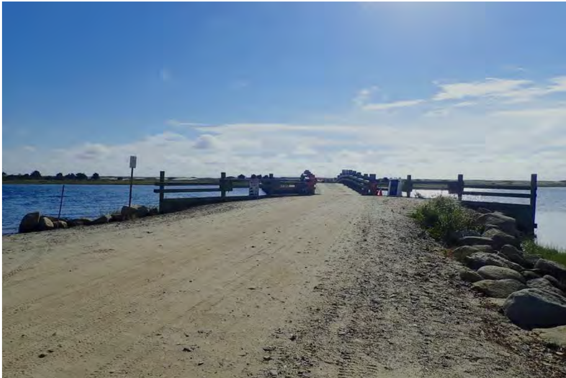
Photo 1: West approach, at-bridge weight posting sign installed at inadequate height.
