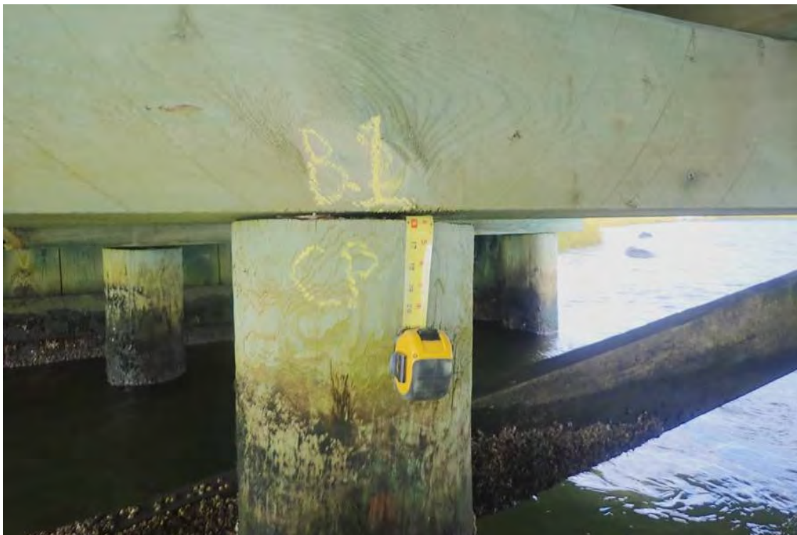
Photo 18: Bent 1 center pile east face, irregular cut off w/ gap between cap.
