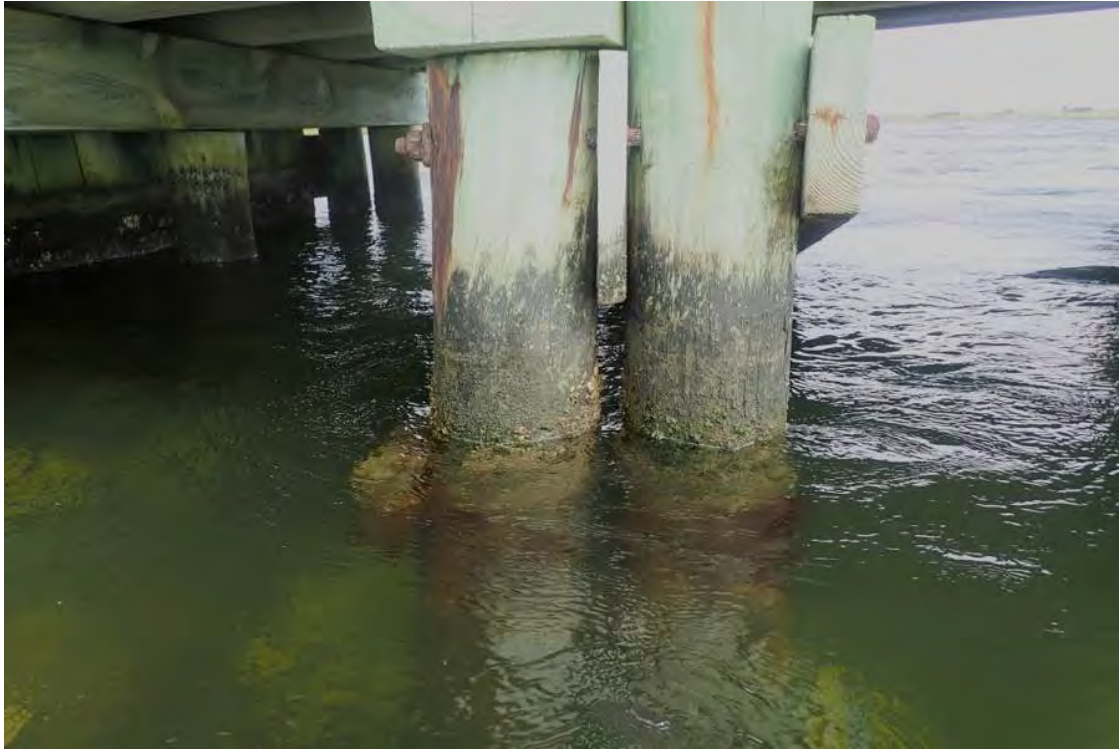
Photo 19: Bent 1 south piles, minor wane w/rust staining.
