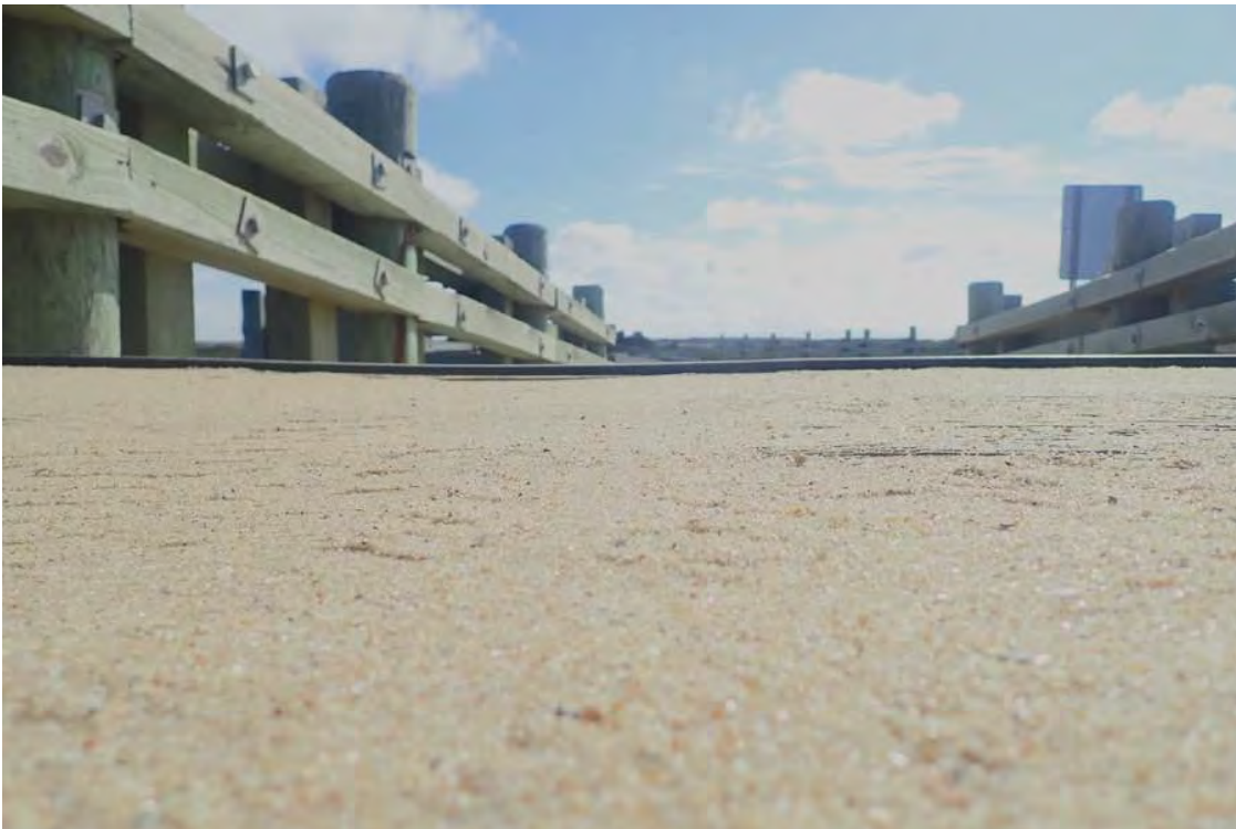
Photo 4: North wheel path looking east (Level @ Bent 4), abraded wheel path w/ sand accumulation & protruding fasteners.
