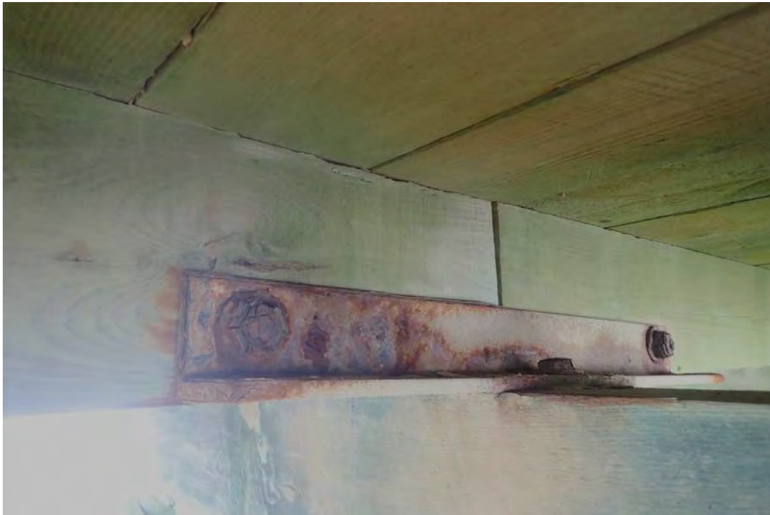
Photo 21: Bent 2 Beam 3 south keeper, corrosion to fastener hardware & angle.
