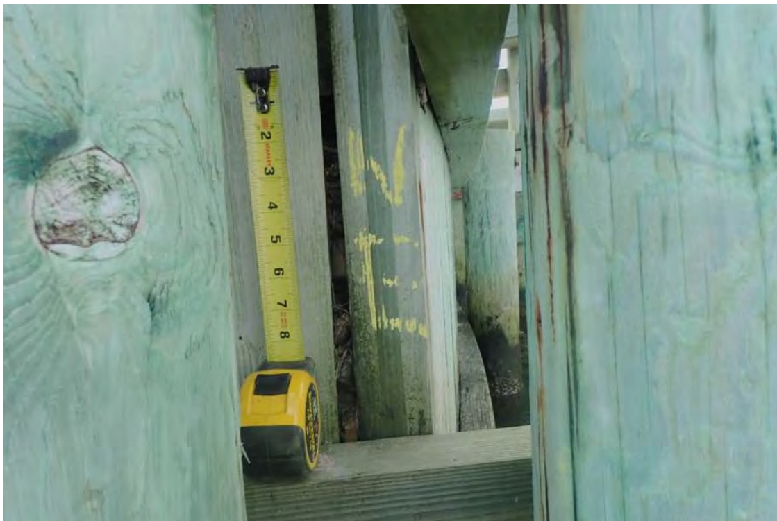
Photo 14: North corner of east abutment bulkhead looking south, bulging/bowing & gap w/ wingwall bulkhead.
