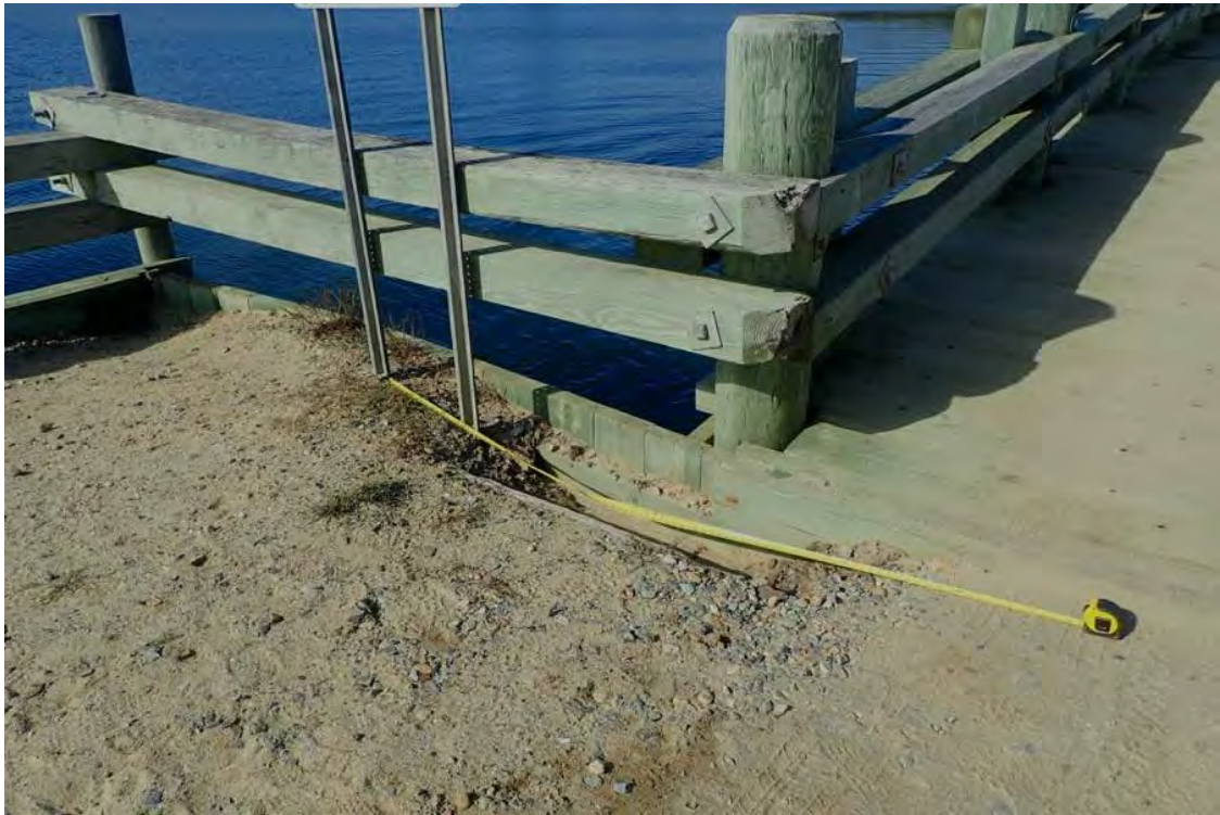
Photo 7: Southeast immediate approach roadway, erosion hole.
