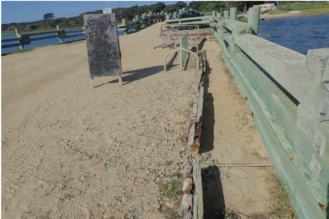
Photo 9: East approach along north wingwall bulkhead, erosion along abandoned bulkhead exposing tiebacks.
