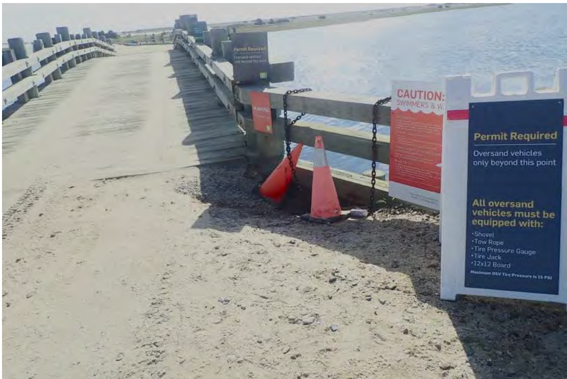
Photo 6: Southwest immediate approach roadway, erosion hole.
