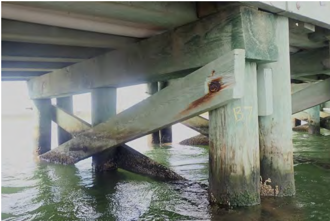
Photo 20: Bent 7 north end of east diagonal bracing, corrosion of fastener hardware.
