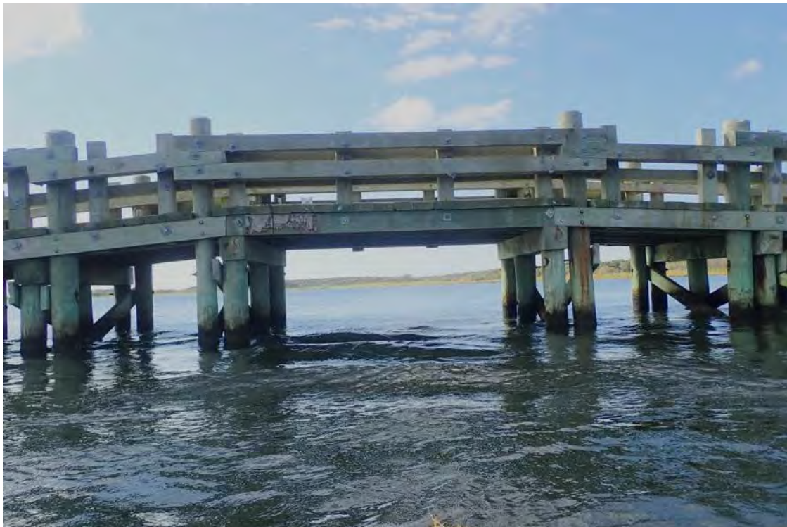
Photo 2: Span 5 north elevation, broken & missing navigation channel indicator sign.
