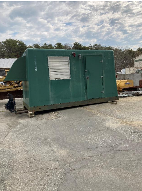
Diesel generator, approx. 850 hrs, worked when removed
