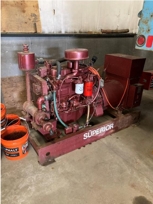
Superior Generator powered by 4 cyl white diesel engine, 202 hrs. Poor condition
