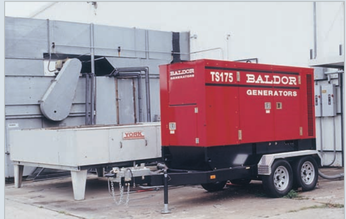
Three Baldor 140kW/175kVA trailer-mounted diesel generators were installed to each of the three 100-ton air conditioning units at our Westville, OK plant. This configuration provided for the reduction of approximately 450 kW of load shaving.
